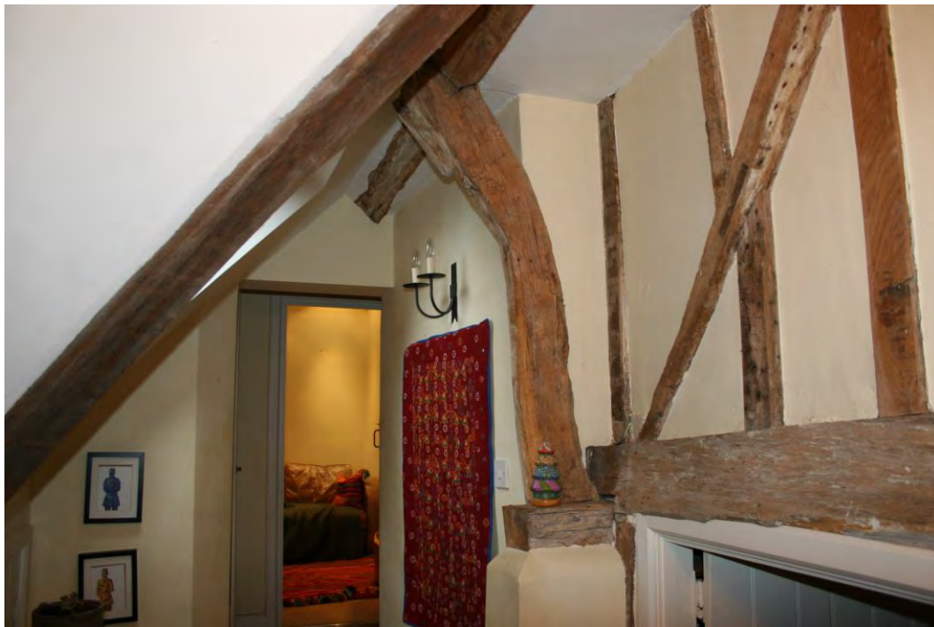
Looking N on the Landing, The cut off top-plate can be seen under the curved shore.
