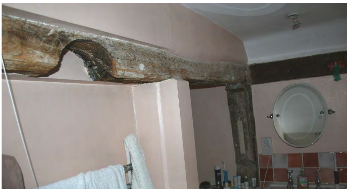
The top plate has a recess for a boiler flue.
