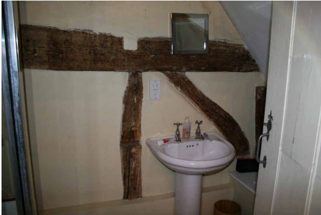
The north end of the tie-beam in the western wall seen in the Bathroom.
