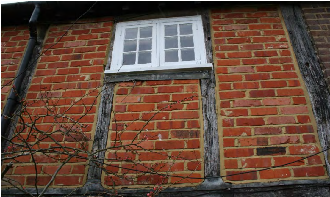
The upper register has LC20th bricks and sandy cement pointing.
