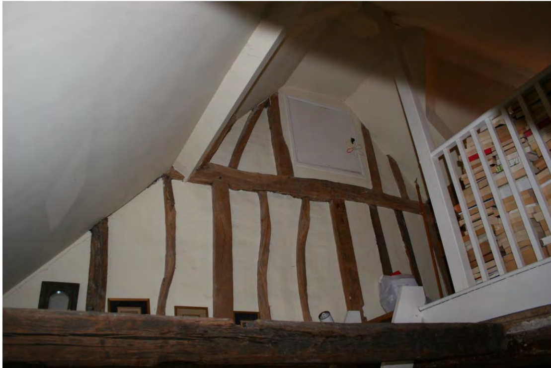
Looking up at the partition wall with the landing. The box frame has added scantling studs.
