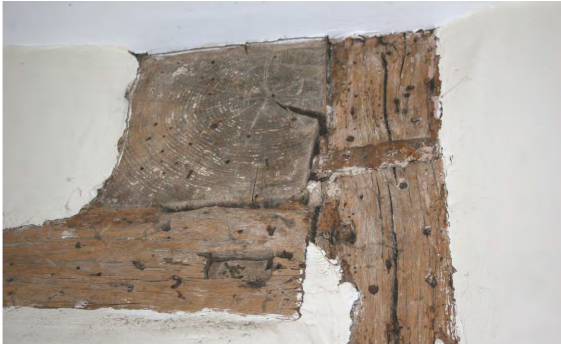
The frame is reinforced with a slender iron joint. Note the sawn off tenon.
