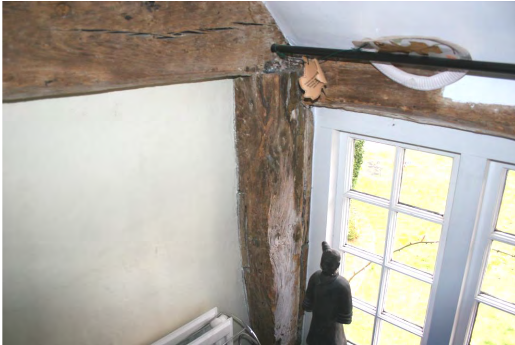
The jowled storey post on the end of the tie-beam in the south wall.
