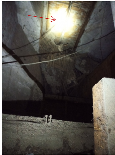
b. Location of the original opening blocked with lath and plaster; collapsed ceiling.
