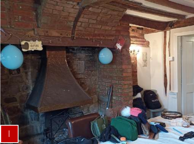
Main house. Dining room. Visible timber frame and C17 plaster decoration around inglenook.
