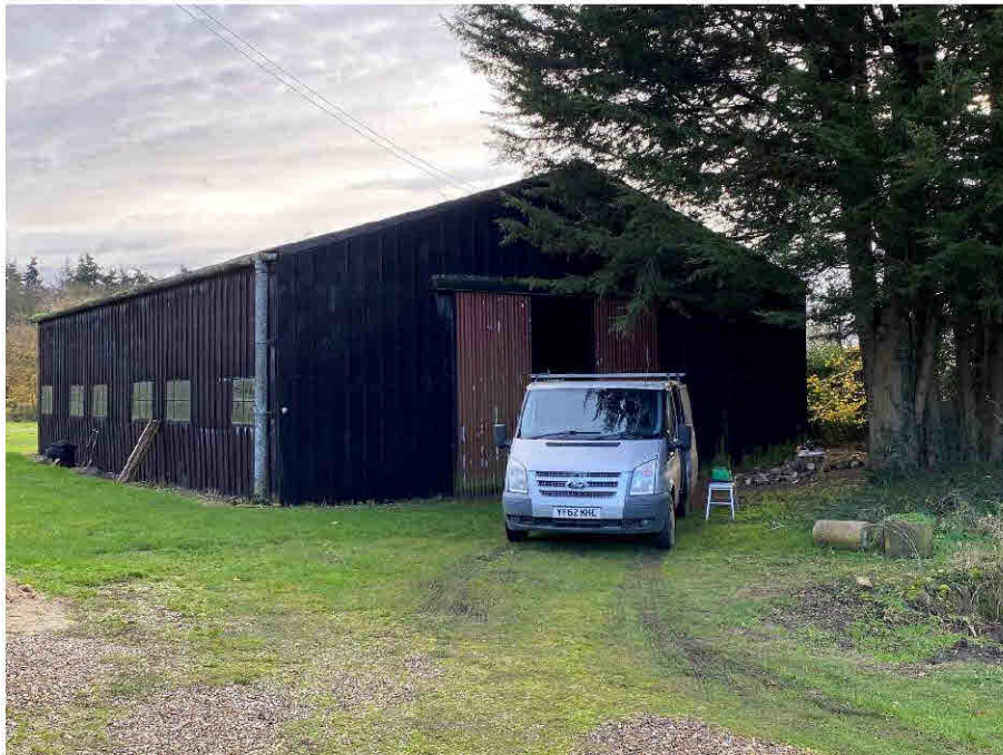
Photograph 1: West Gable Elevation and North Flanking Wall, Note Proximity of Mature Fir Trees.
