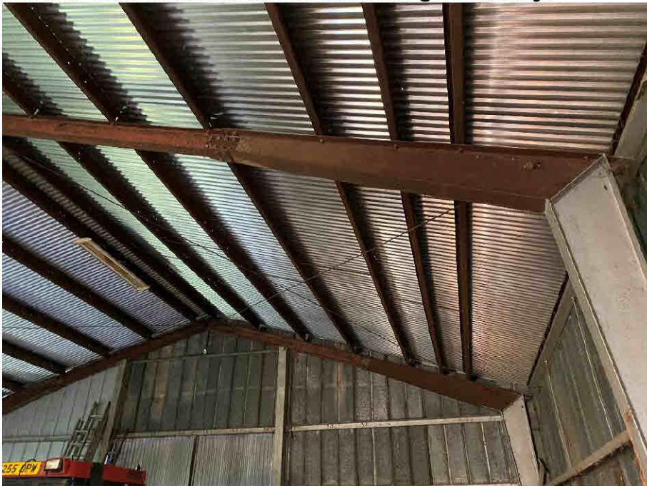
Photograph 3: Typical Portal Frame, Note Welded Mitre Joint at Eaves and Cover Plate Splice Connection Further up Rafter.
