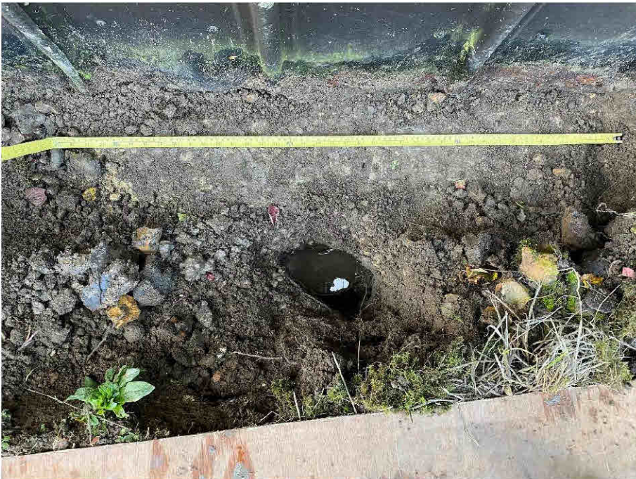
Photograph 17: Trial Hole Exposing Edge of Concrete Pad Foundation. Pad Width Measured at Approximately 900mm.
