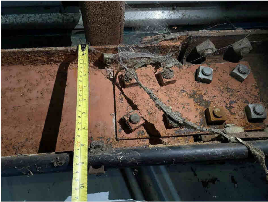
Photograph 6: Close Up of Cover Plate Splice Connection to Rafter. Note Surface Corrosion to Steelwork. Rafter Depth Approx. 200mm.
