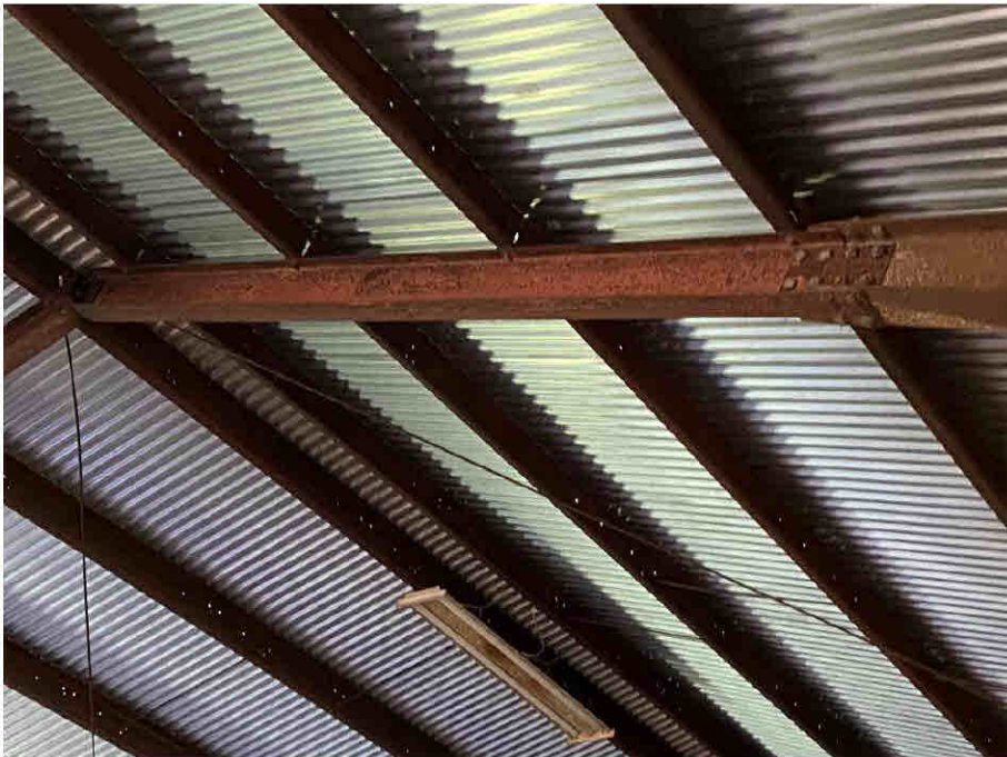
Photograph 5: Typical Portal Frame Rafter. Note Apex Section of Rafter is Not Tapered.
