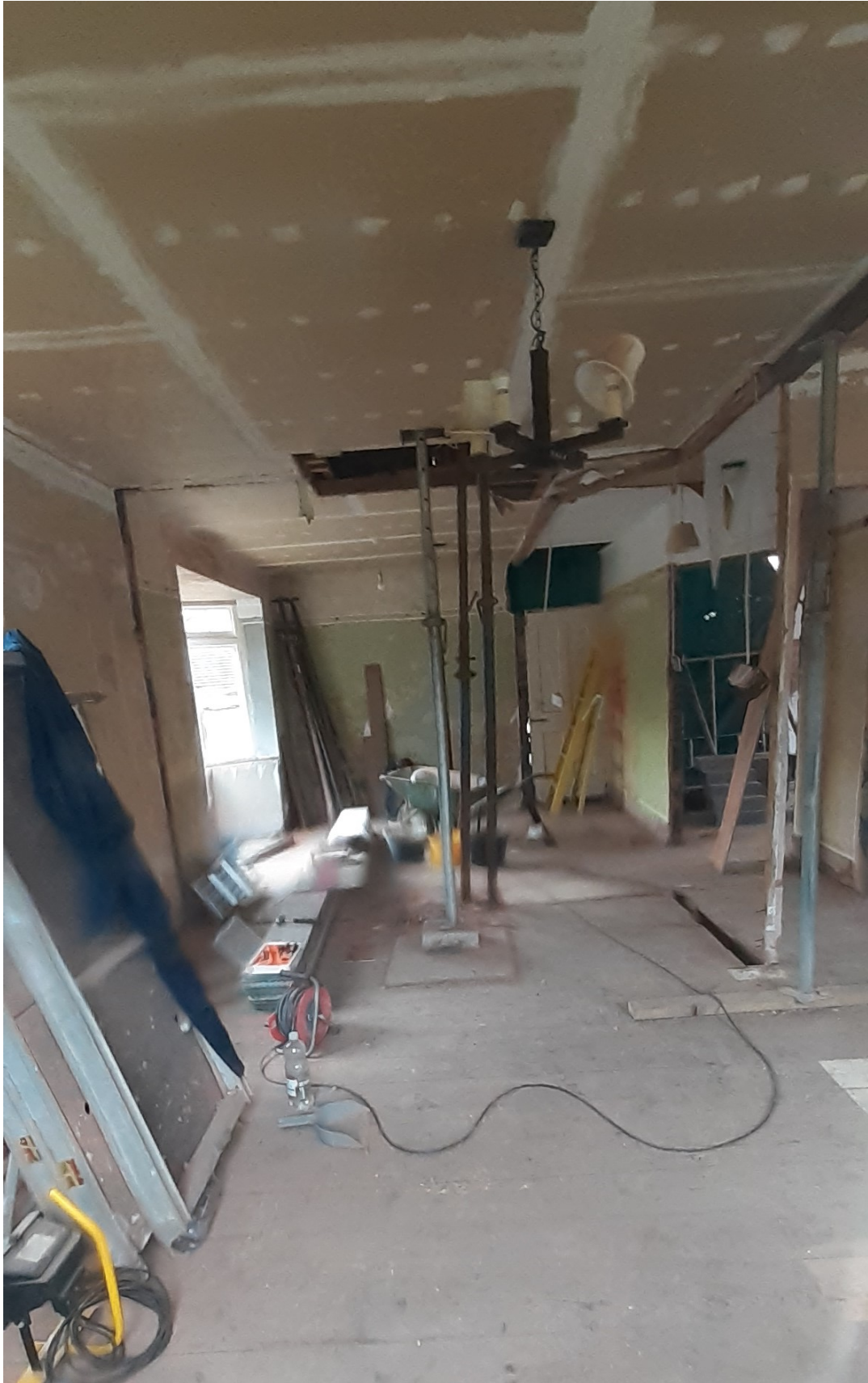
Internal view showing chimney breast and internal walls removed between living room and bedroom.
