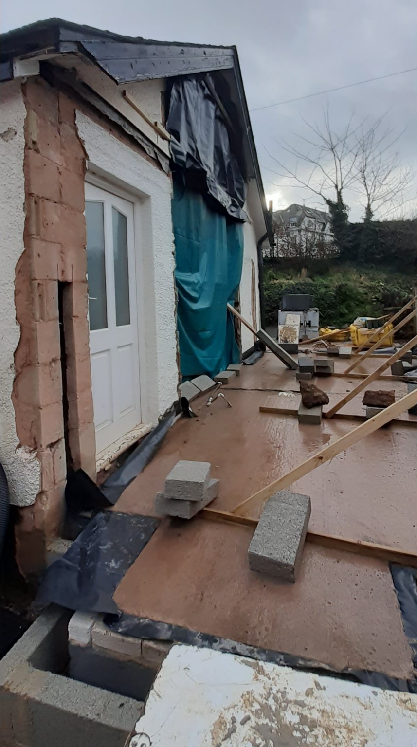
Rear elevation showing construction works for the rear extension (23/0764/FUL) including new footings, below ground drainage, external walls, and concrete floor slab.
