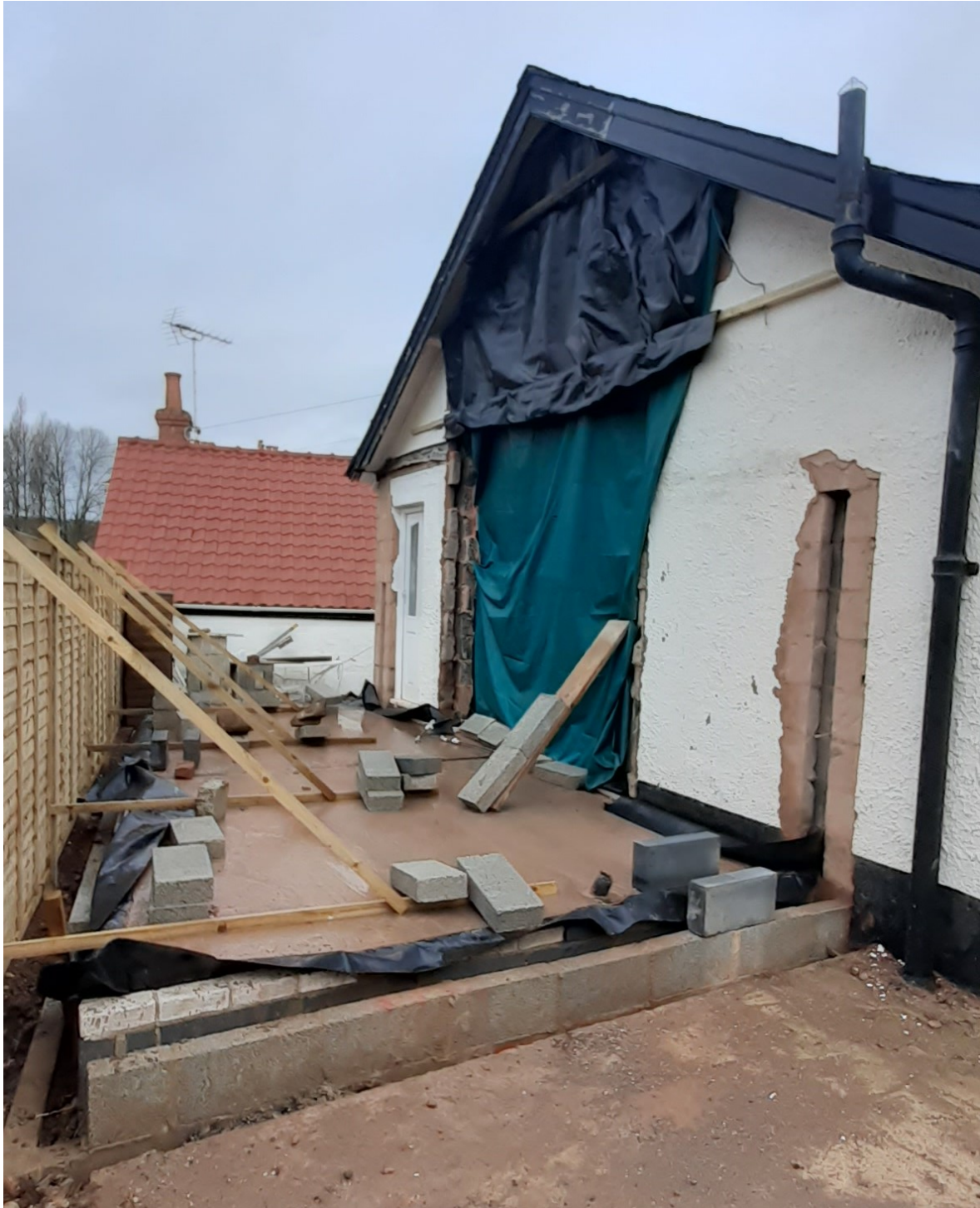
Rear elevation showing construction works for the rear extension (23/0764/FUL) including new footings, below ground drainage, external walls, and concrete floor slab.
