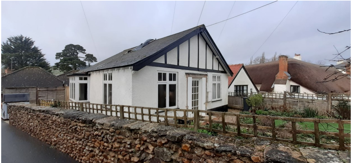
Street elevation facing Hillside Road, Sidmouth, showing porch and chimney stack demolished.
