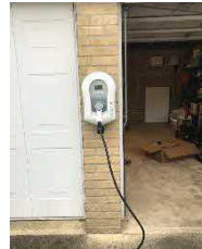
Battery System EV Charging Point
