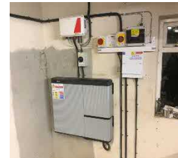
SolarEdge LG chem Zappi 2
