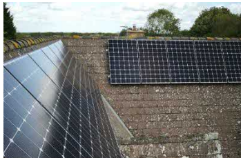
Solar PV System 7.35 kW Solar Panels LG35U
