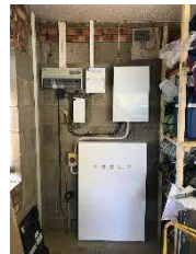
Battery System Solar Inverter
