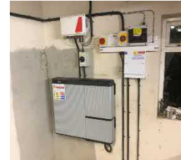
SolarEdge LG chem Zappi 2
