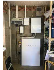
Battery System Solar Inverter
