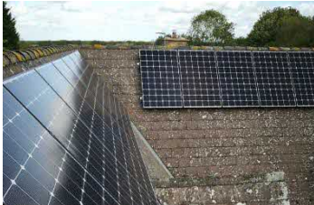
Solar PV System 7.35 kW Solar Panels LG35U
