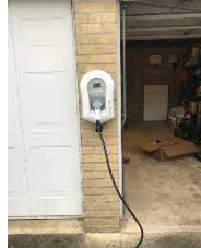
Battery System EV Charging Point
