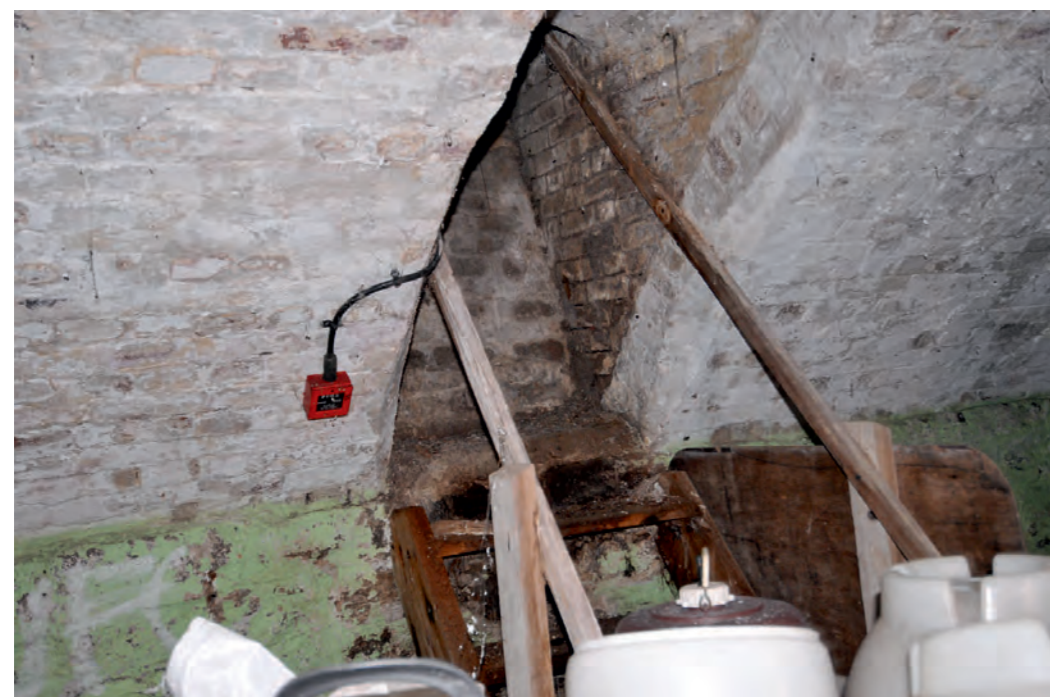
Blocked former entrance
