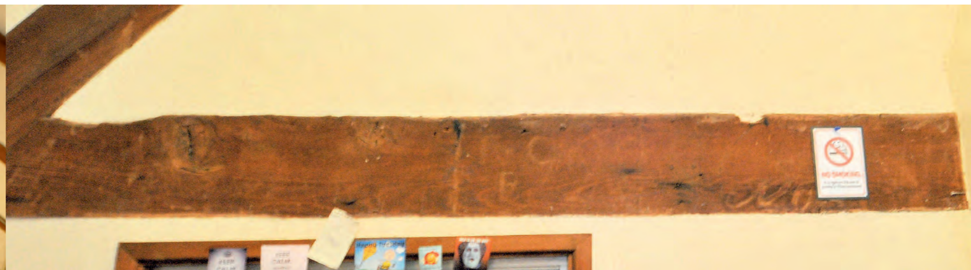
Detail of 19th C. inscription on tie beam
