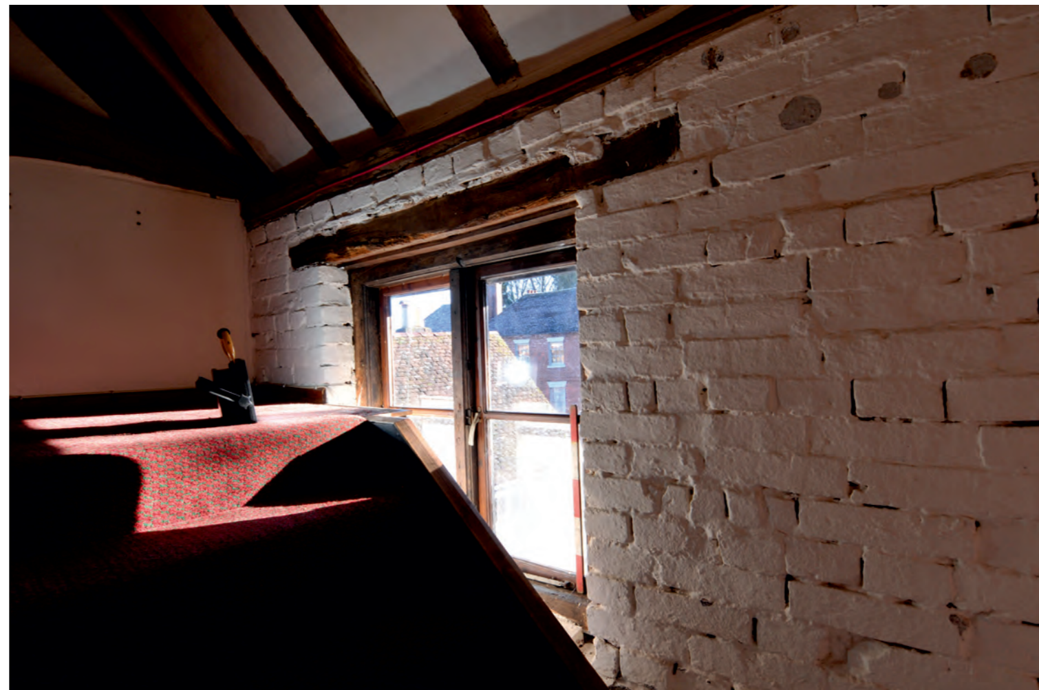
Probably original early 19th C wooden casement window frame, replaced side opening casements
