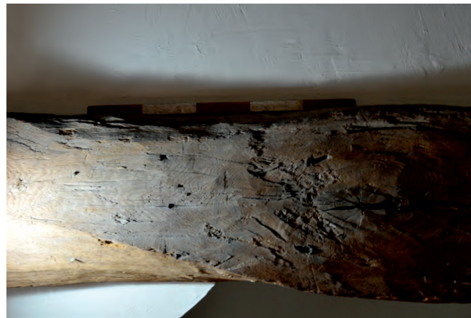
Truss 1 Scar of strap hanger
