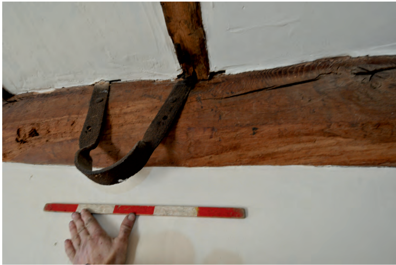
First floor Strap hanger
