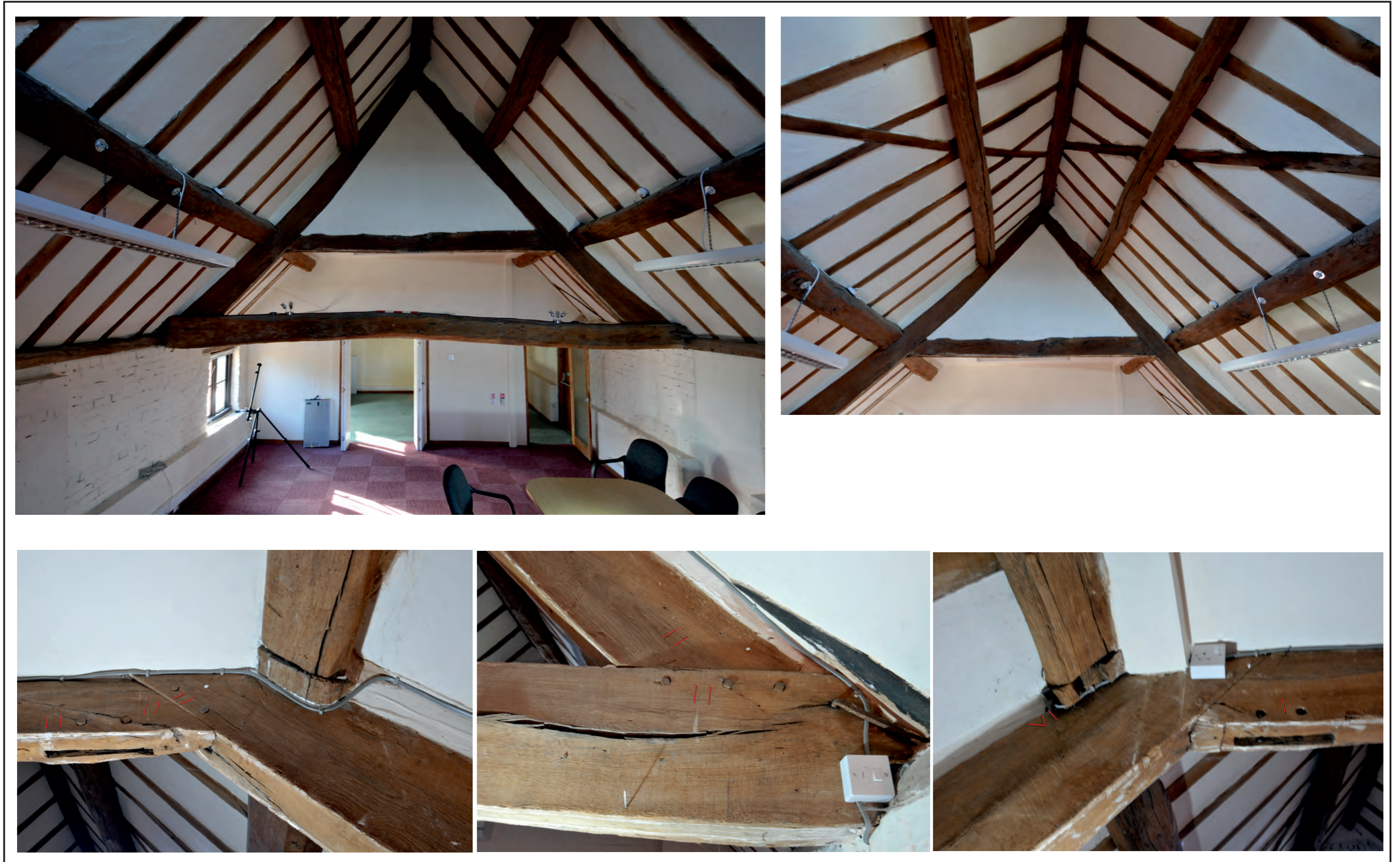
Figure 12: Truss 2, with details of assembly marks on western face. Note that the queen strut mortices on the collar have no corresponding mortice on the tie beam.
