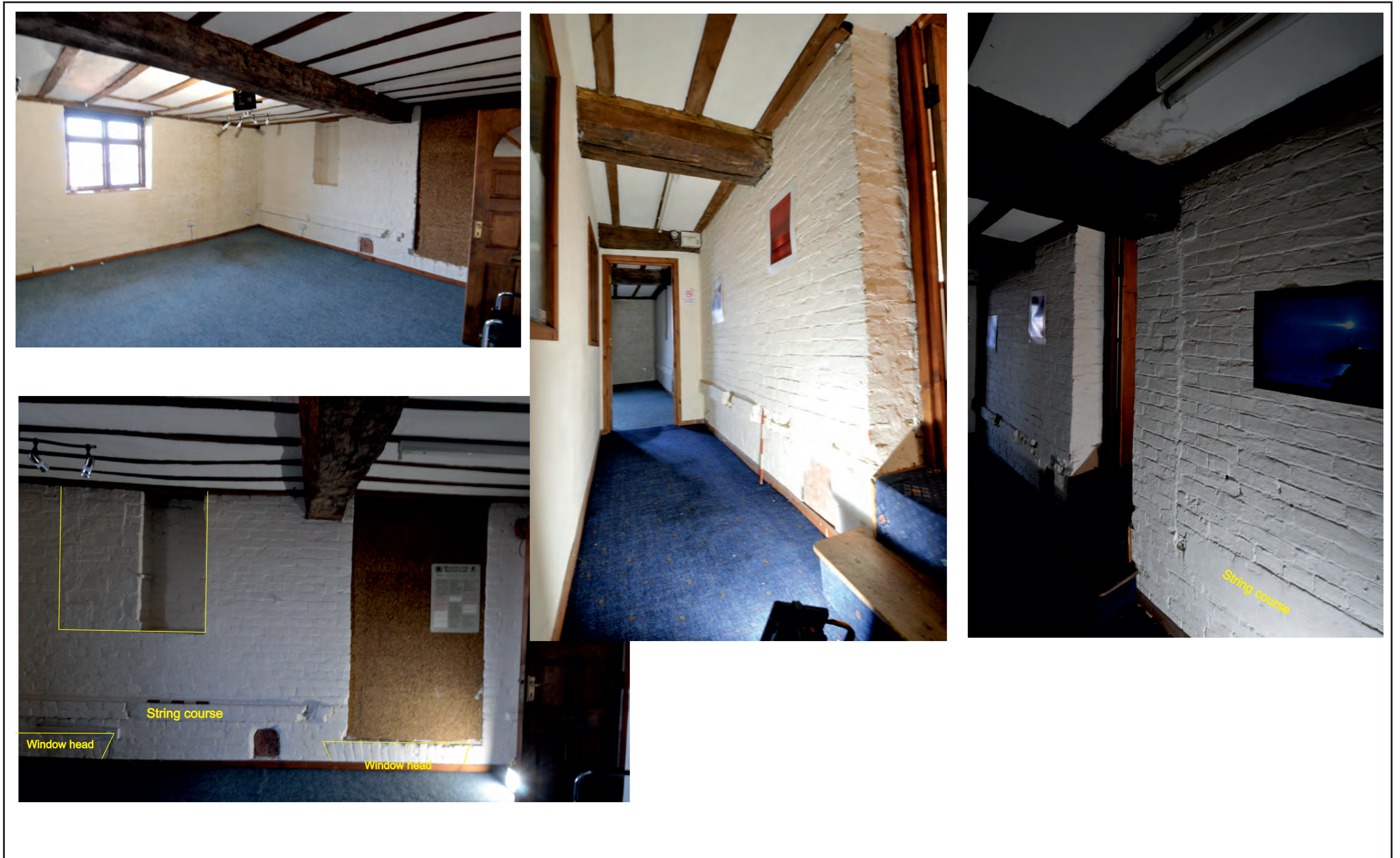
Figure 13: Northern wall of Block 1, visible from within Block 2, showing former string course and heads of blocked ground floor north facing windows
