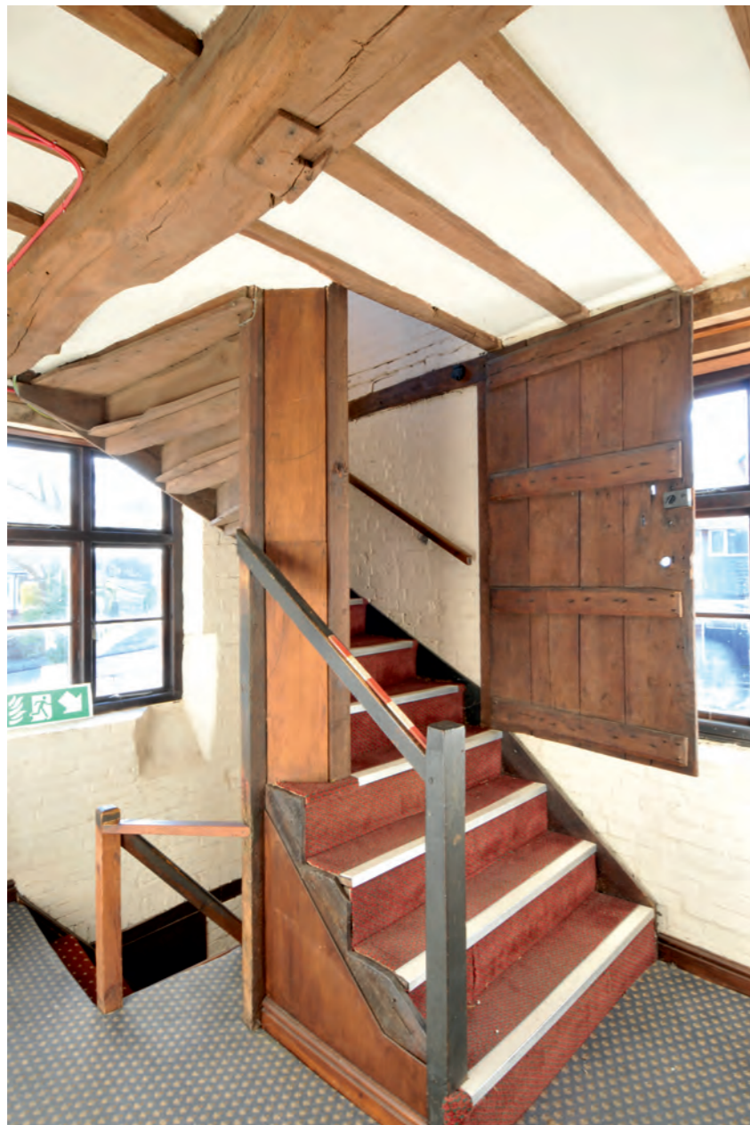
Stair at first floor level, with rehung door from elsewhere in the building
