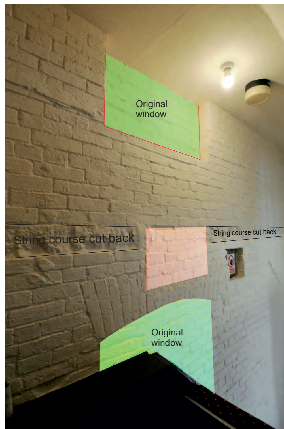
Ground floor window head and sill of 1st floor blocked window openings of Block 1
