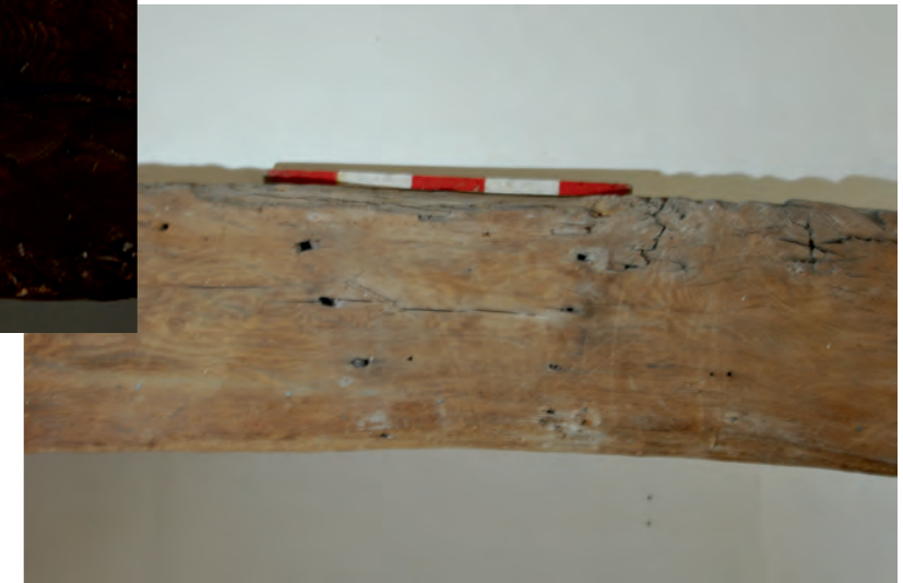
Truss 1 Scar of strap hanger
