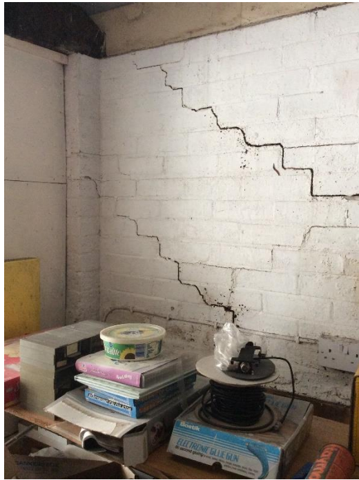
Cracks to right flank wall
