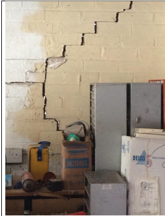
Cracks to right flank wall
