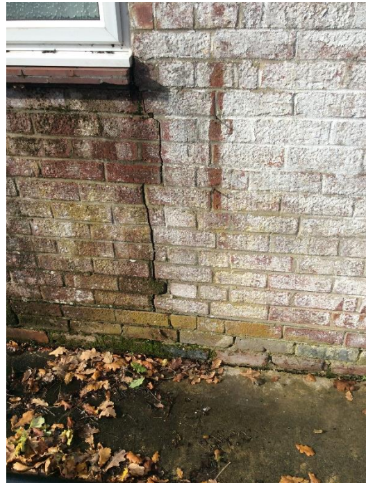
Crack to rear wall
