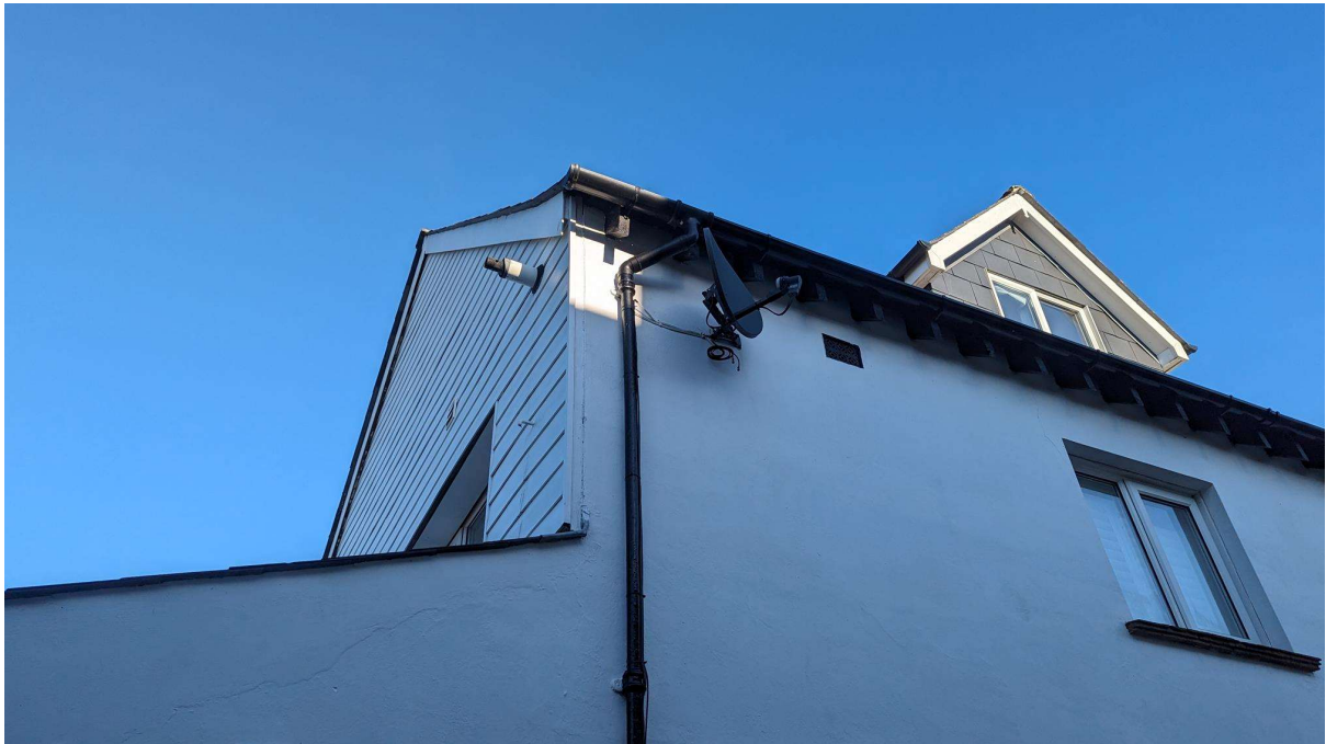
Photo7– View of the Area of dwelling proposed for attachment, with no gaps in eaves or gable.
