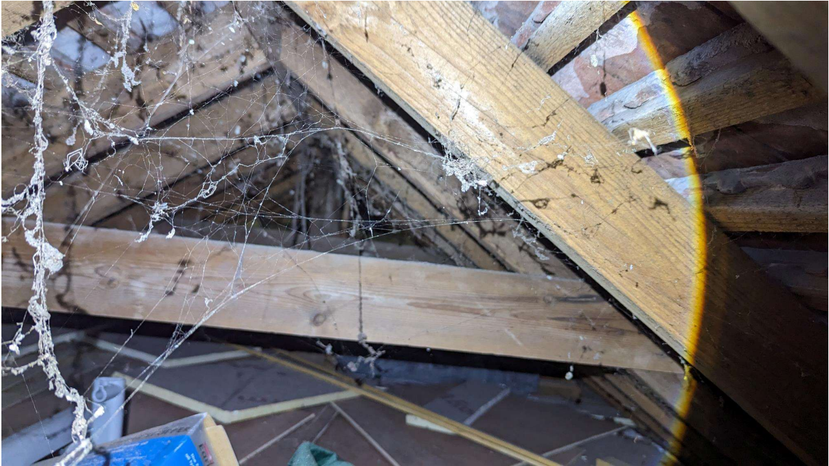
Photo 5 – View of the Unconverted roof above the middle portion of the garage.
