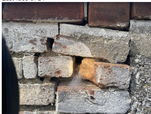
Holes in brickwork leading into cavities
