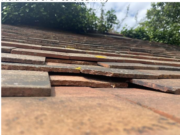
Broken roof tiles. Roof is lined beneath.
