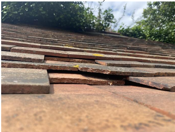
Broken roof tiles. Roof is lined beneath.
