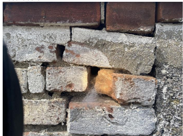
Holes in brickwork leading into cavities
