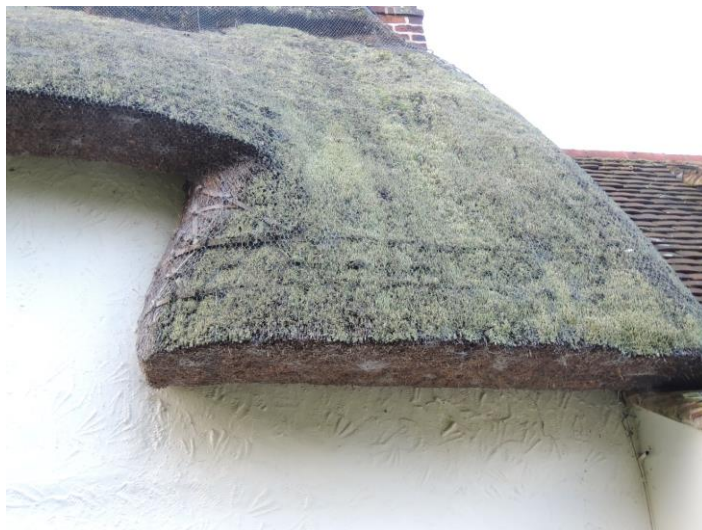
Photo 8: The adjacent thatched roof is covered with mesh to deter birds and rodents and, by default, bats
