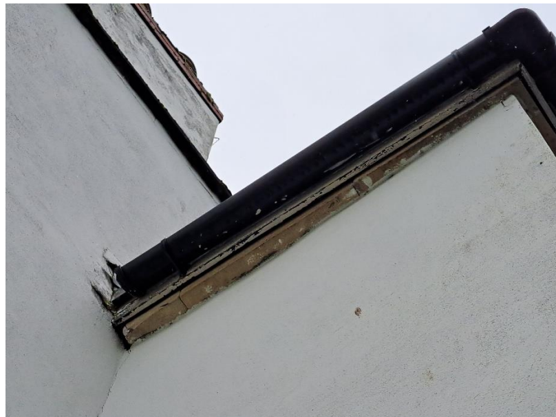
Large hole at junction of external wall and linear gaps between fascia board and stonework on west elevation
