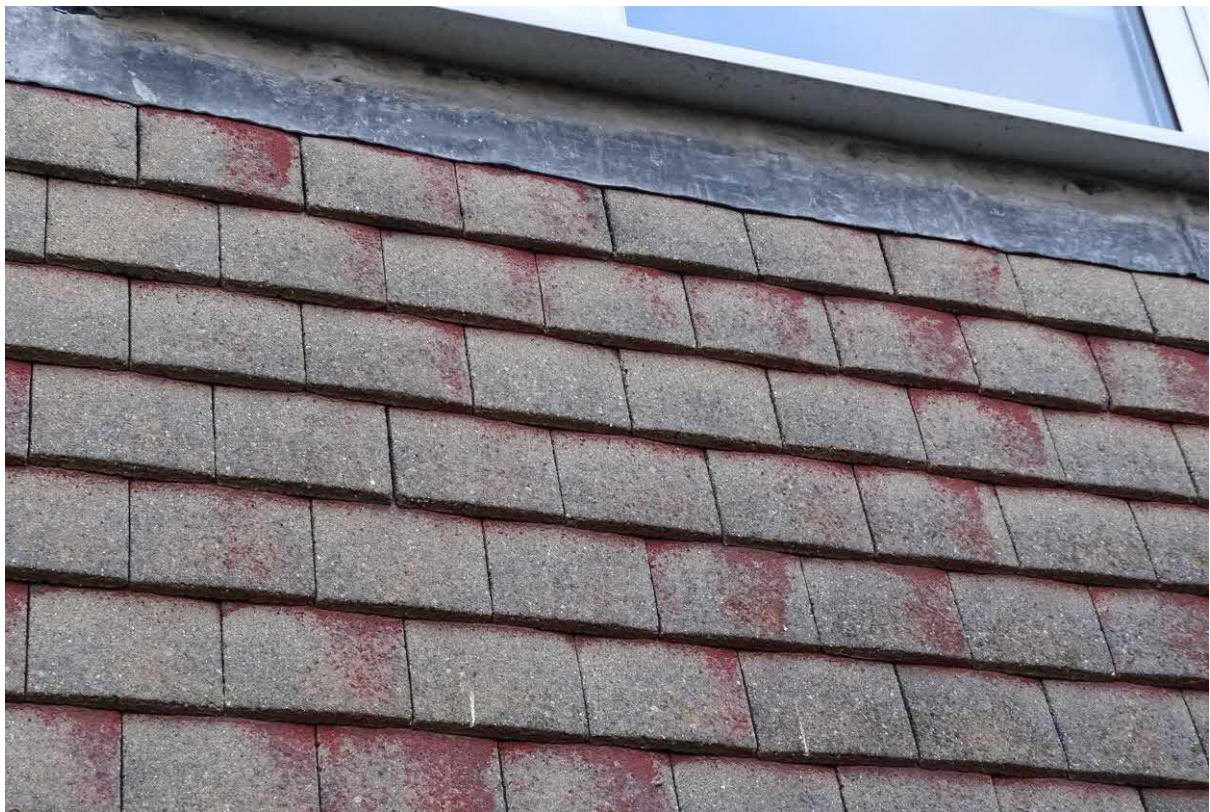
Image 4 – Close view of vertical hanging tiles to rear of property to demonstrate condition
