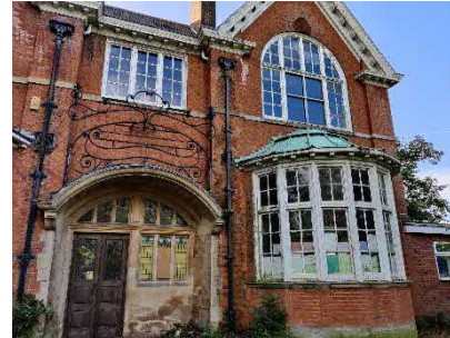
B4 western elevation with smashed windows and belfry
