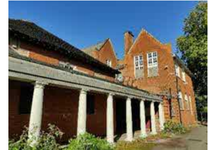
B5 slipped tiles hanging tiles also western elevation
