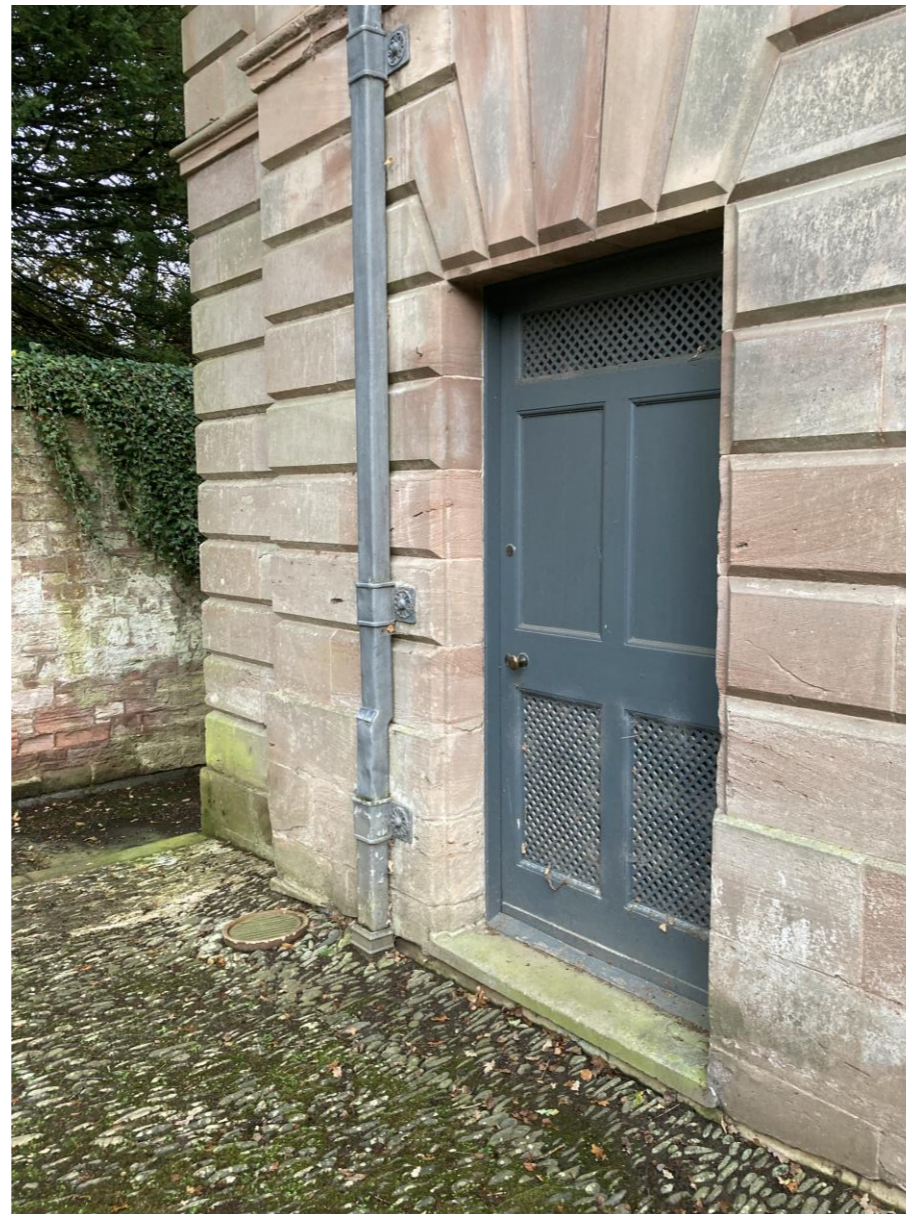
Fig. 13 External door to north west gable illustrating diamond head voussoirs, cobbles and adjustment to lower door panels.
