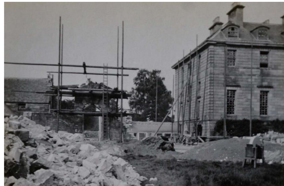
Fig. 08 Enabling works as part of the 1913-16 works prior to the removal of the lateral wall to form the new wing
