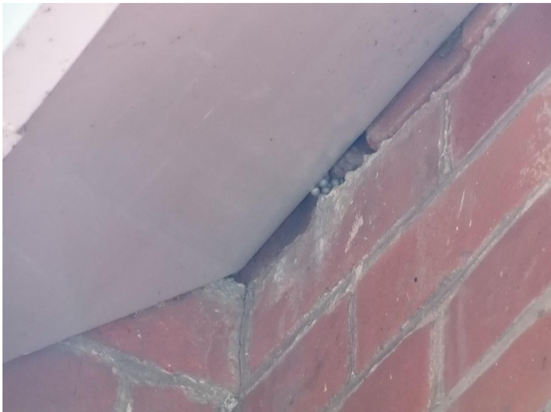
Photo 8 , crevice between soffit box and brick wall on the south aspect.
