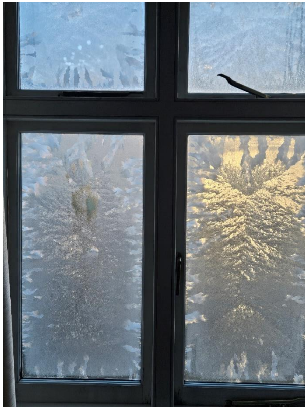
Image taken on 18/01/2024 showing frost on the glass of first floor west facing window.
