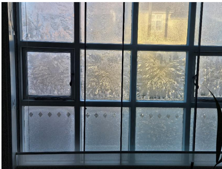
Image taken on 18/01/2024 showing frost on the glass of ground floor west facing window.
