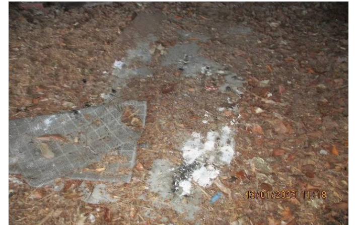
Photo 6: Splashing found on the centre floor of 'Building 3'.
