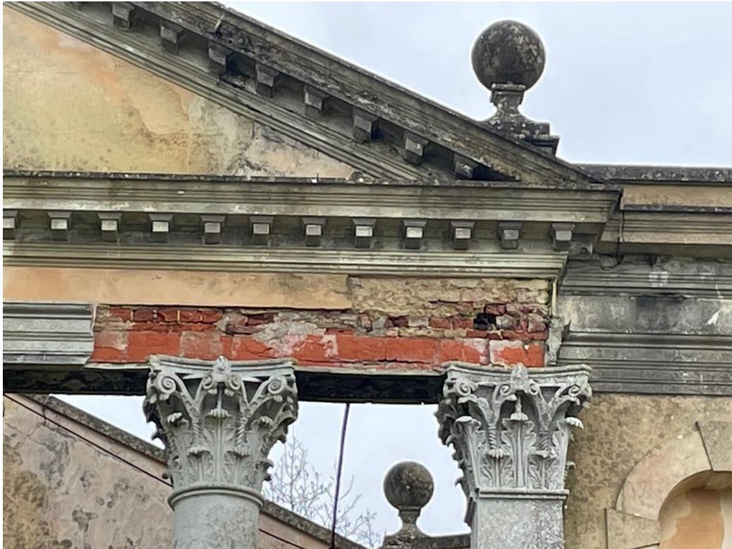
Close up of collapsed string and brick substrate
