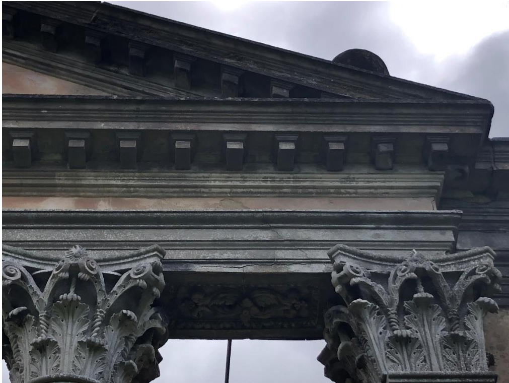
Adjacent cracking to render
