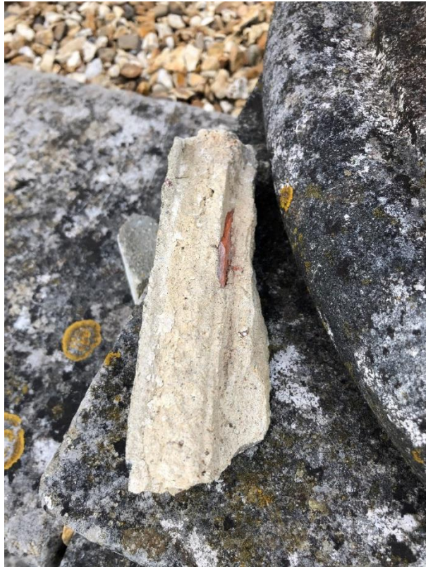
Fallen piece of render and brick substrate at ground level
