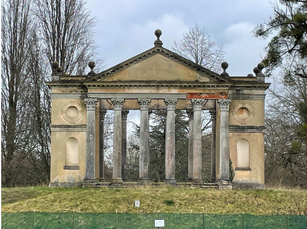
General view December 2023 showing collapsed section of string
