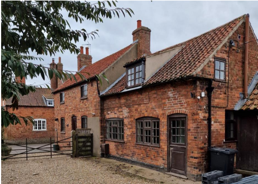
Photograph showing the existing ground floor windows and door to be replaced
