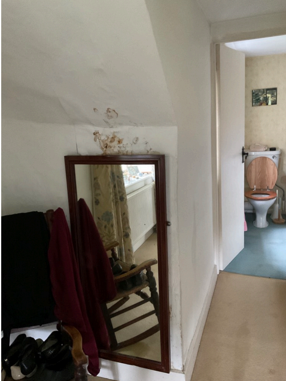
Water ingress under back left corner of flat roof, wetting roof frame and witchert wall fabric.
