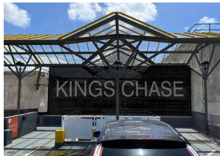
View from MSCP first floor deck - perforated panel screening railing and services
