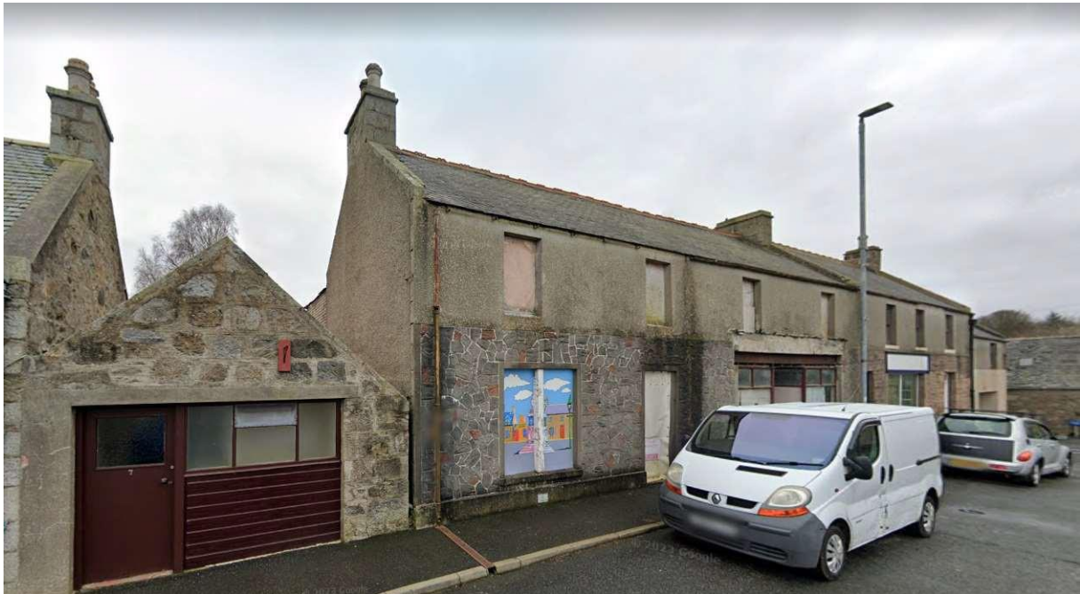
Above: Google Streetview images c.2023 showing window openings boarded up & missing chimney cans.
