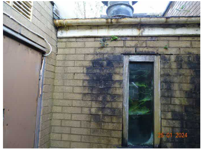
Photo 8 – Office structure front elevation showing rotten window, dark staining, corroded gutters, vegetation above – door to Bank main building on the left hand side.
