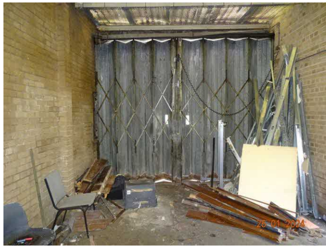
Photo 9 – Garage structure interior – front area showing folding steel vehicle door & steel angle purlins spanning across.
