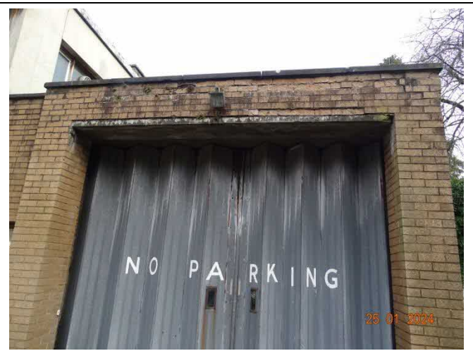
Photo 4 – Front elevation showing piers to side of vehicle door & masonry over shallow r.c. lintel.
