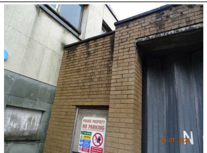
Photo 6 – Link wall viewed externally showing door to enclosed area and dark staining below copings.
