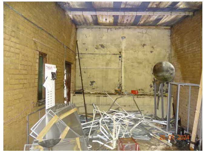
Photo 10 – Garage structure interior – rear area showing upper & lower rear retaining wall – internal door & window to Office structure on left hand side.
