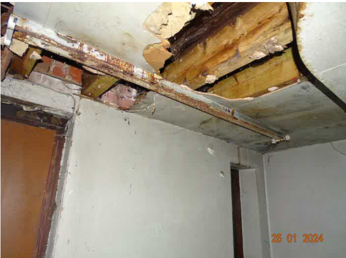
Photo 12 – Office structure interior showing failed roof structure.
