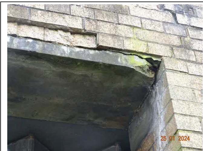
Photo 5 – Partially failed bearing of vehicle door lintel at right hand side pier.
