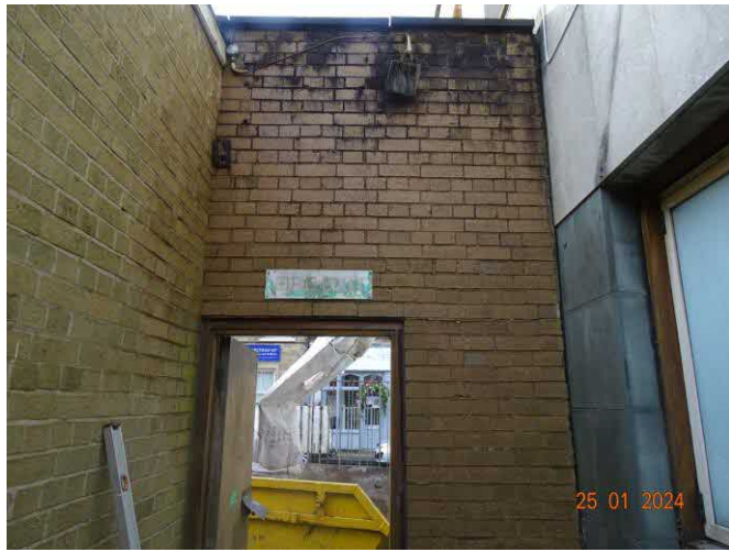
Photo 7 – Link wall viewed internally with corroded bracket near junction to Garage left side wall and gap to Bank main building on right hand edge.
