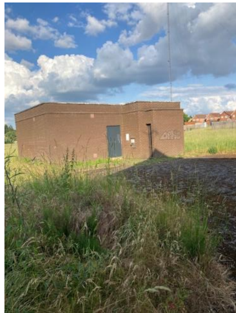
Figure 8. Substation building, view from north west. Internal access was not possible at the time of the survey.
