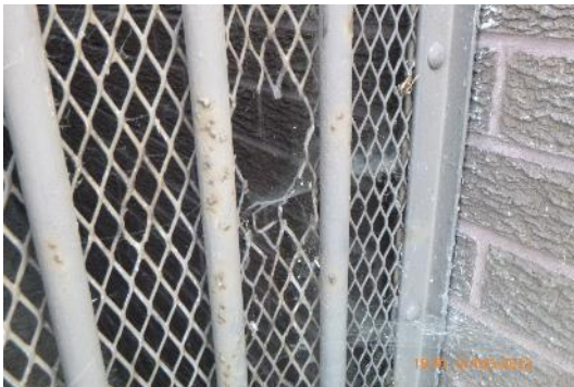
Figure 3. Hole in the grate (cobwebbed over).
