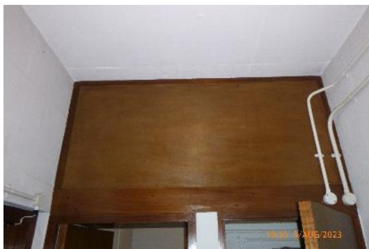
Figure 9. Internal inspection above small closet not possible due to lack of an access hatch.
