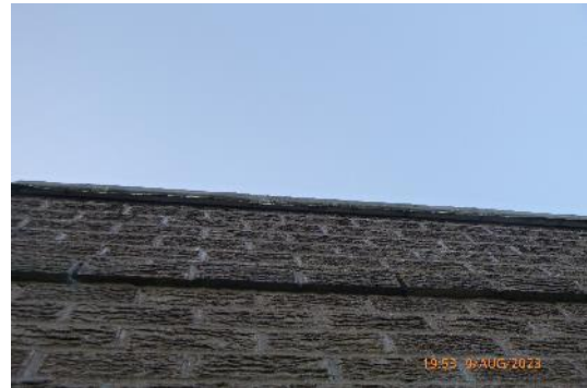
Figure 2. Roof cap has warped slightly, possibly creating small (<10mm) gaps.
