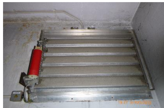
Figure 6. Internal view of vent on eastern elevation (closed and cobwebbed over).
