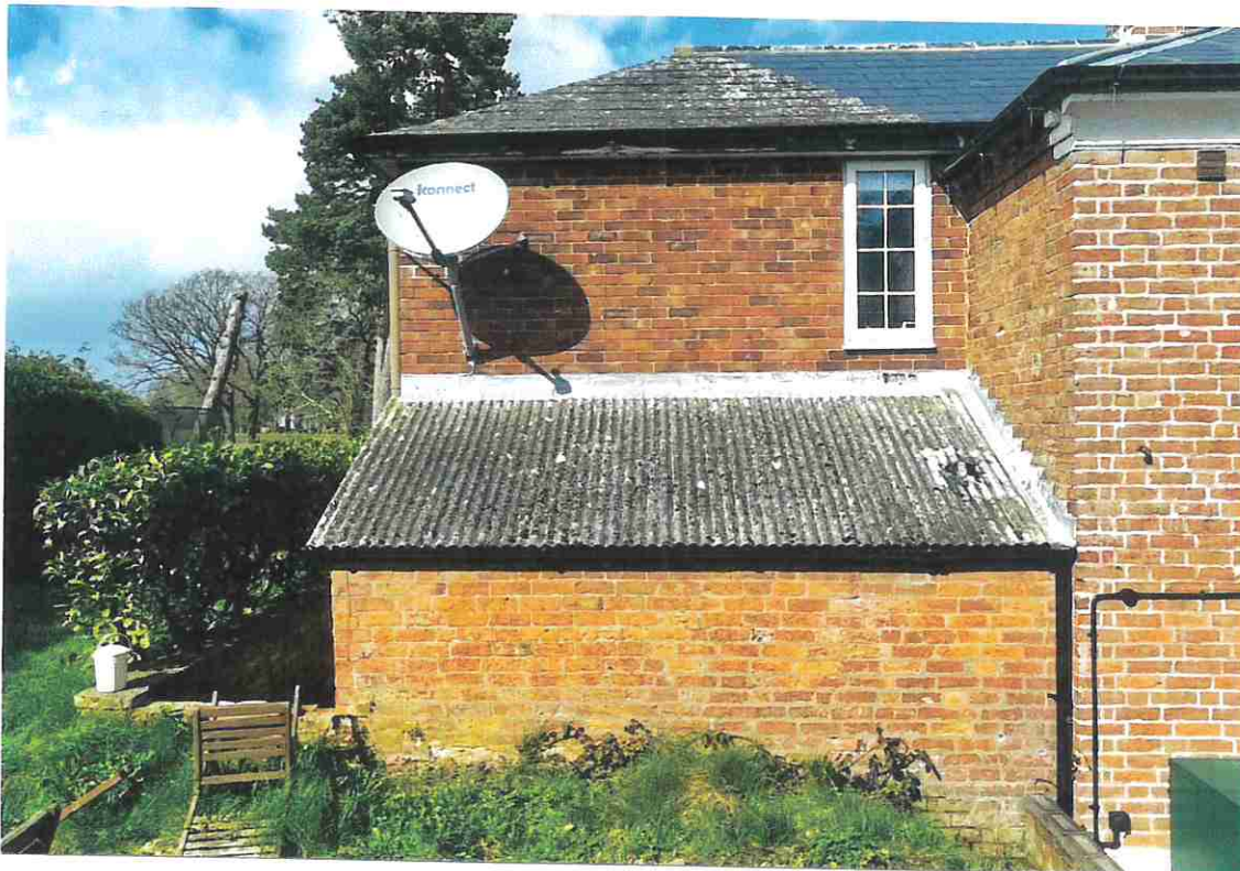
PHOTOGRAPH 9 - DETAIL OF THE OLD LEAN TO WHICH IT IS PROPOSED TO RAISE IN HEIGHT TO HELP COVER THE EARLIER REAR EXTENSION WHICH DOESN'T MATCH THE ORIGINAL HOUSE.
