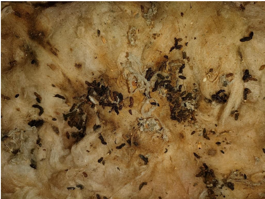
Plate 8: Bat droppings in roof void, brown long-eared bat.
