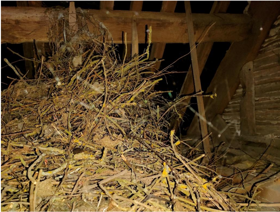
Plate 9: Jackdaw nest in roof void.
