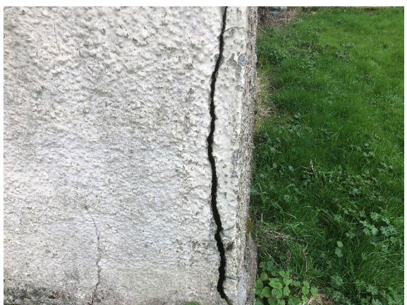
Cracks to walls at ground level.
