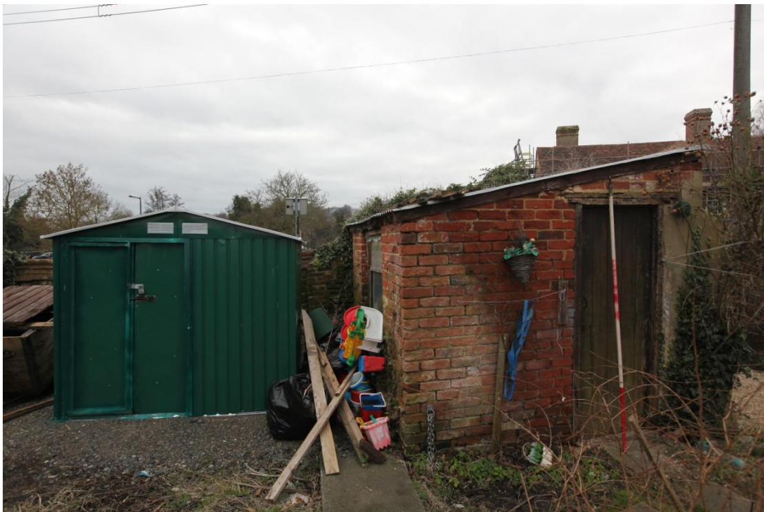
Illus. 22. The roadside wall from the garden of no. 12 to the east showing the mid-20 th century shed that was not present in 1924 (figure 6). The poorly built walls of the shed consist entirely of stretchers and are presumably only 4.5 inches thick, but the interior was inaccessible at the time of inspection.
