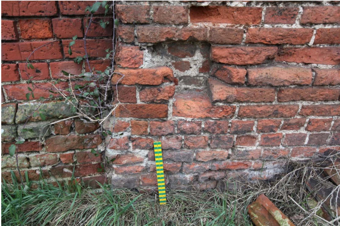
Illus. 15. A detail of a damaged but once neatly cut and ostensibly original recess in the earliest section of wall (1) at bottom left in illustration 14. Such recesses are usually associated with horizontal locking bars, but it is difficult to see how a doorway could have projected at this point.
