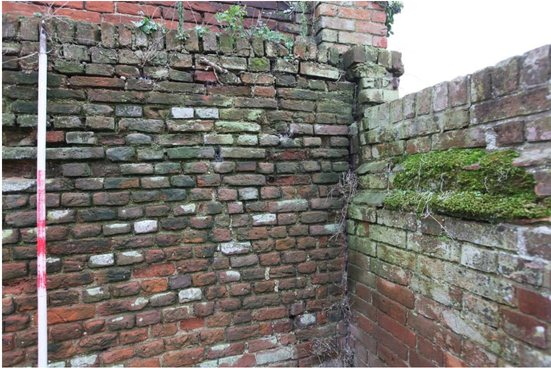
Illus. 21. A detail of the probably 19 th century but possibly 18 th century garden wall in illustration 20 (8) showing the closers or quarter bricks that respect its right-hand edge where it directly abuts the oldest 16 th or 17 th century section of the roadside wall (1). This edge remains vertical and no gap has opened against the earlier wall, indicating that the latter's lean has not increased since the addition of the buttress.
