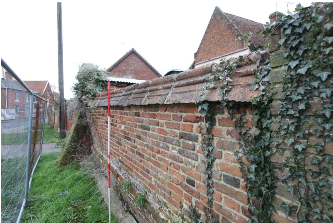
Illus. 10. The rebuilt section of wall from the south (5) showing its slight lean supported by the buttress and caused by the weight of the 20 th century garden shed and the much higher ground in the garden to the east (producing a differential of some 0.75 m).
