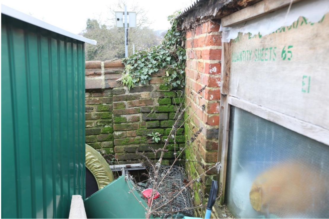
Illus. 23. The eastern side of the roadside wall in illustration 22 showing the vertical step in its face that coincides with the recently rebuilt section (5) to the left.
