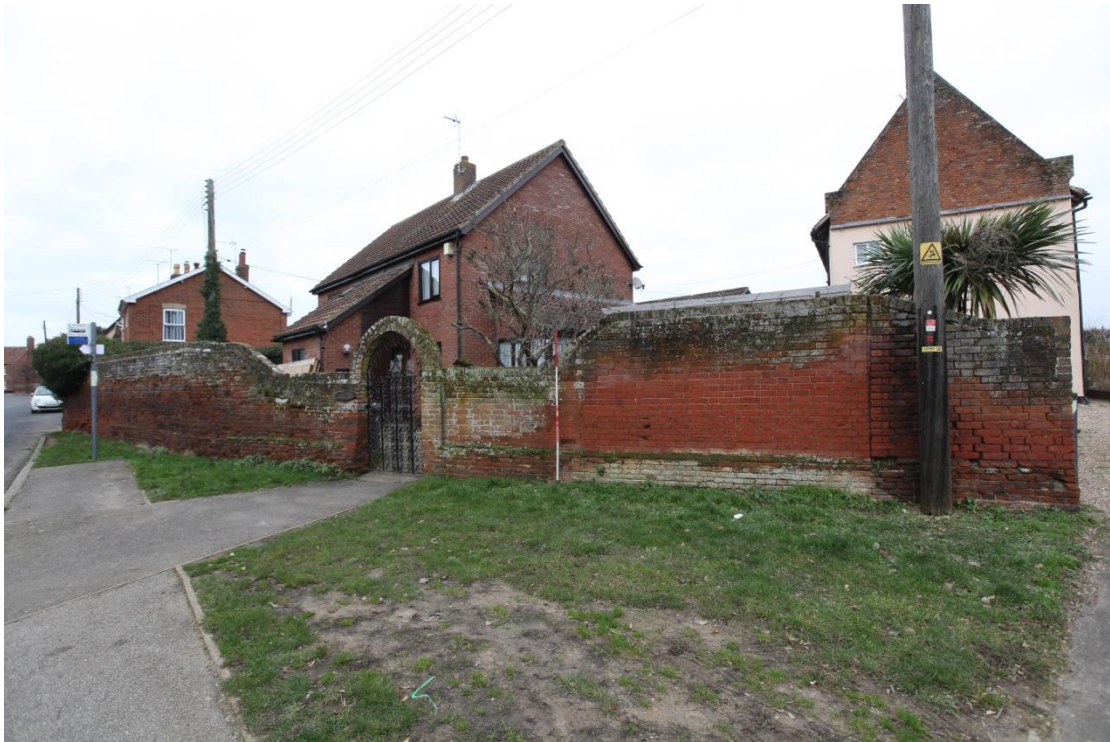
Illus. 27. The northern end of the roadside wall from the triangular section of waste ground showing the straight vertical joint between the surviving gable of the mid-19 th century pantiled shed to the left of the telegraph pole and the yard wall of no. 12 to the right. Although structurally distinct these walls are almost identical and clearly contemporary or almost contemporary. The right-hand edge of the yard wall is respected by closers and adjoined a gate from the outset (although the entrance may have been less wide than today as the opposite edge in illustration 16 has been rebuilt).
