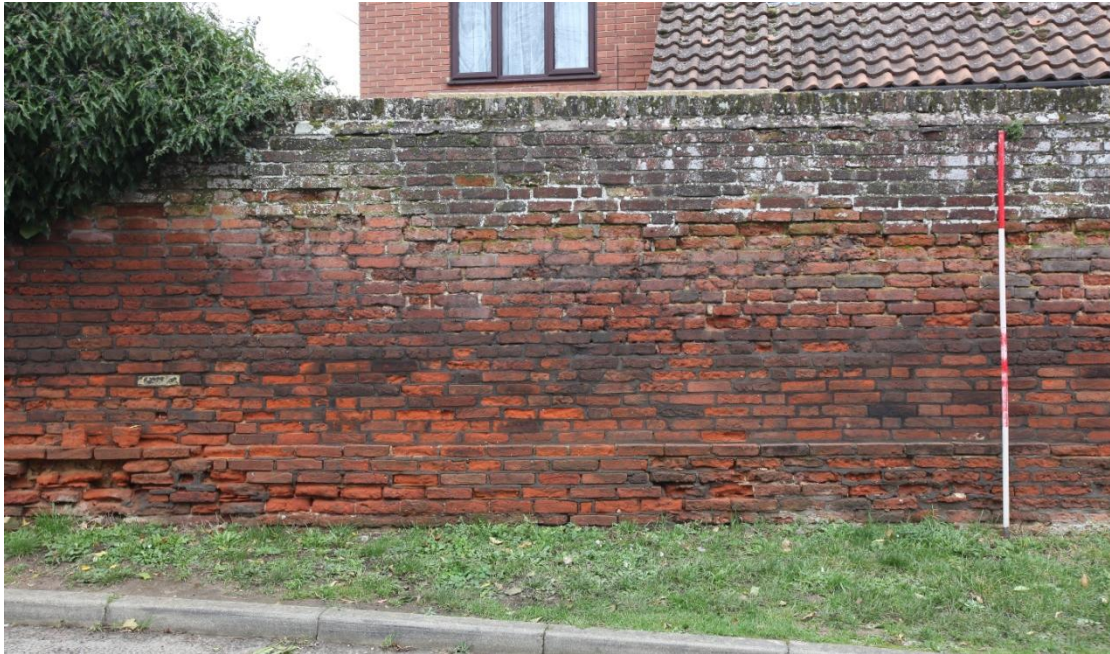
Illus. 7. The roadside wall of River View consists of similar narrow bricks to those of 12-16 Bridge Street, but the bonding differs and it was probably rebuilt as part of the new animal yard in the 19 th century. The plinth lacks chamfered plinth bricks and consists chiefly of stretchers while the rest is a random mixture of bonds. It has been heavily repointed and partly rebuilt using a hard cement mortar which has exacerbated the process of decay.
