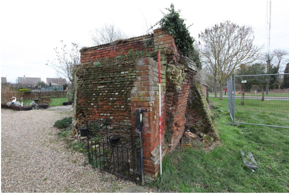
Illus. 17. The historic wall from the entrance to no. 12 to the north-west, showing the 19 th century boundary wall (8) overtopped by the 20 th century shed (7) on the left. The 16 th or 17 th century wall (1) is leaning outwards relative to the vertical 19 th century section in the foreground, but the 19 th century buttress is evidently doing its job as no further movement seems to have occurred since its construction. The recent damage to its top corner has been caused by the ostensibly new corner pier of the 20 th century shed which has been built directly above.
