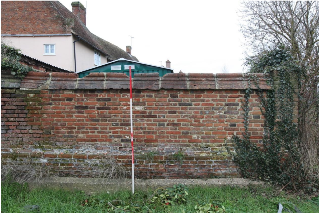
Illus. 9. A detail of the southern section of the wall in illustration 8 which has been entirely rebuilt in recent years using a patchwork of re-used bricks laid in a light-coloured cement mortar imitating lime (section 5 in figure 12). The terminal pilaster to the right is also modern, but the plinth survives at least from the 19 th century and consists of stretchers with a single course of headers below the plinth. The coping tiles have also been re-used.
