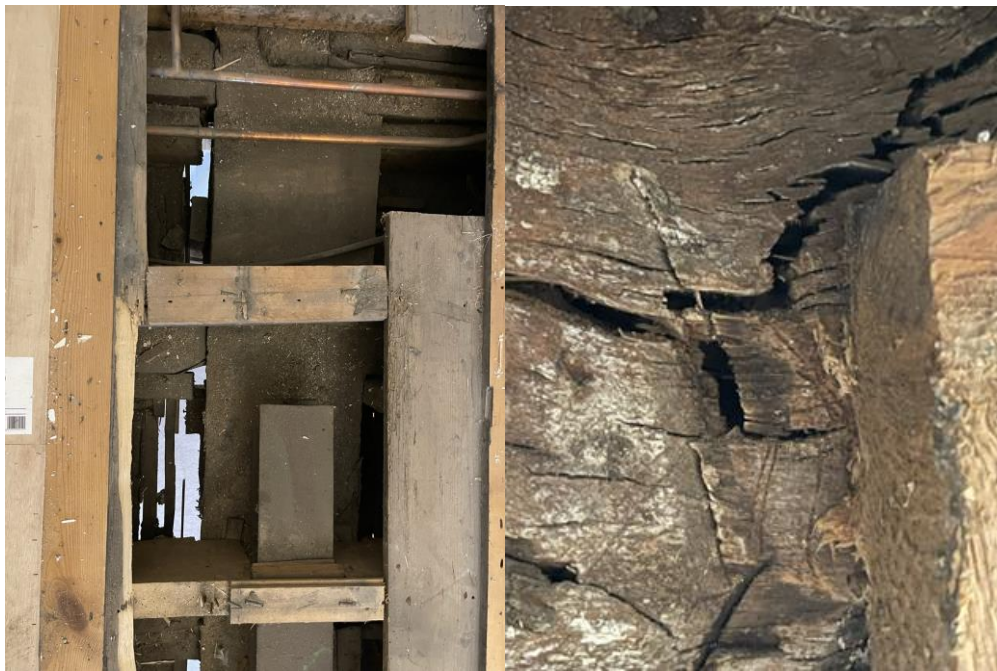
Fig. 9: Exposed structural beam showing previous repair
