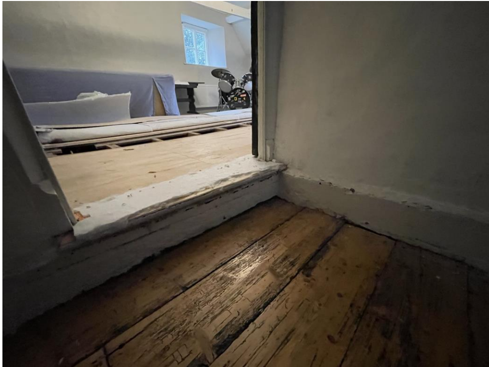
Fig. 8: Second floor door threshold showing change in floor level
