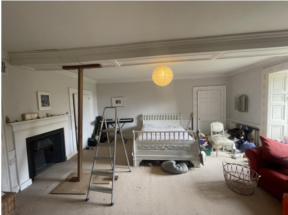
Fig. 6: First Floor bedroom showing temporary propping
