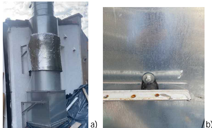
Figure 3 Evidences of the extraction system serving Bento House with use of a) acoustic noise reduction blanket and b) anti-vibration mounts
