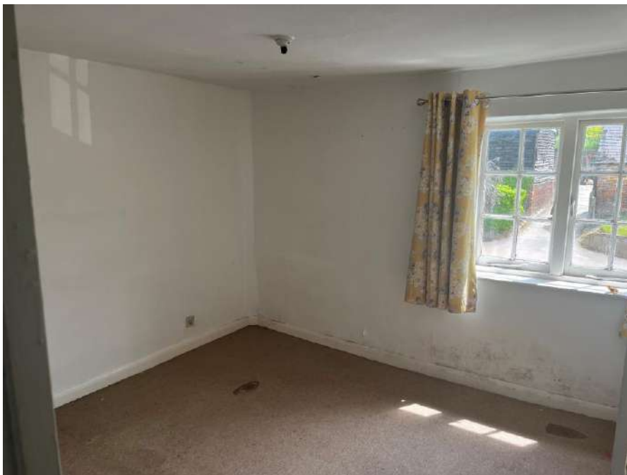
View from the first floor bedroom to no.9 showing the front wall and front window
