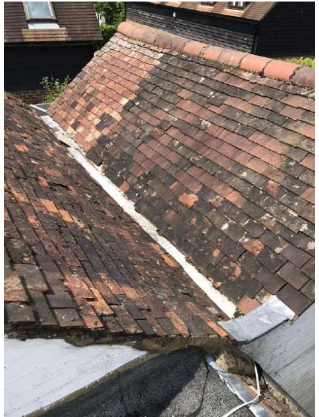
View from the outer lead valley gutter to no.5 between the two dual pitched roofs.
