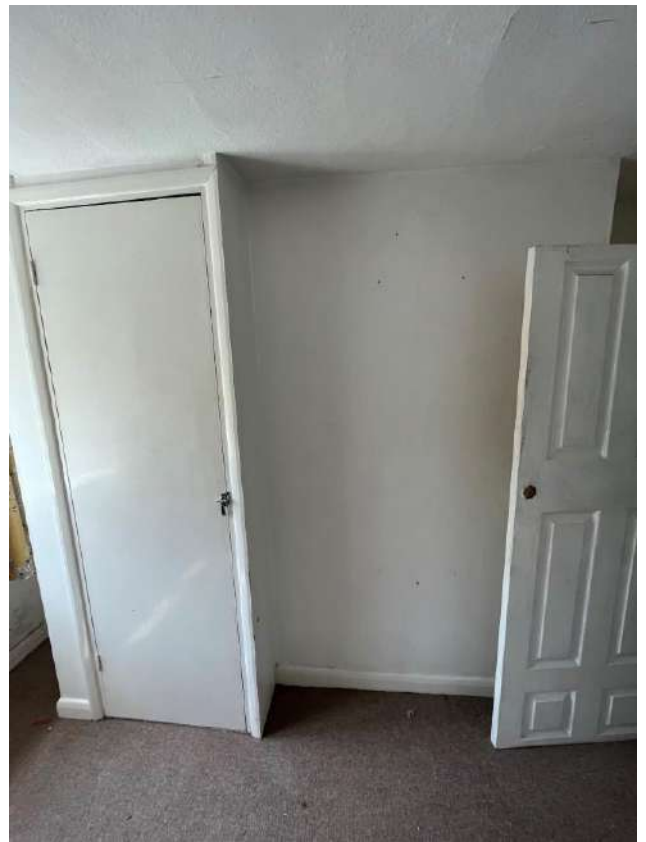
View from the first floor bedroom to no.9 showing the store cupboard and door.
