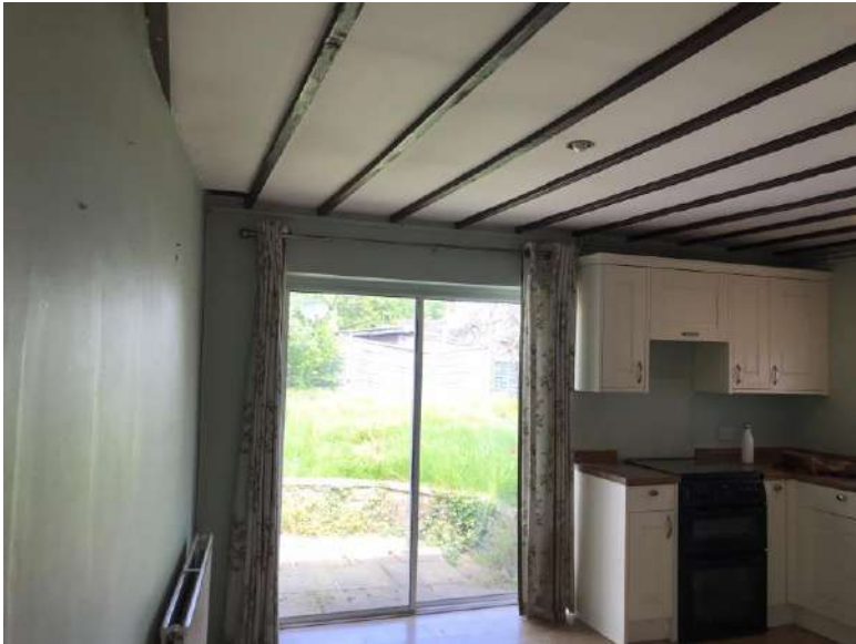
View of the rear kitchen straddling the back of both dwellings. The ceiling is plasterboard with exposed rafters that have been stained.
