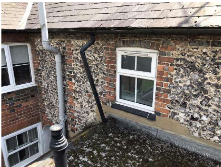
Closer view of the Upvc casement window to the bathroom to no.9, along with the external drainage and boiler flue.
