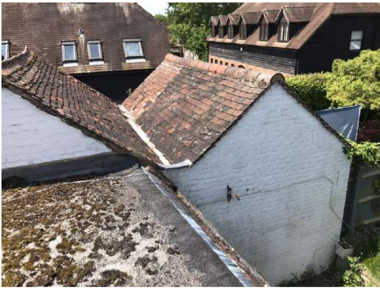
View from the site's rear extension roof towards the flanking wall to the rear extension to no.5
