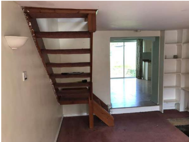
Internal view taken from the ground floor lounge to no.7 looking towards the back and showing the timber stair with its open treads and the opening in the rear wall leading to the kitchen extension.
