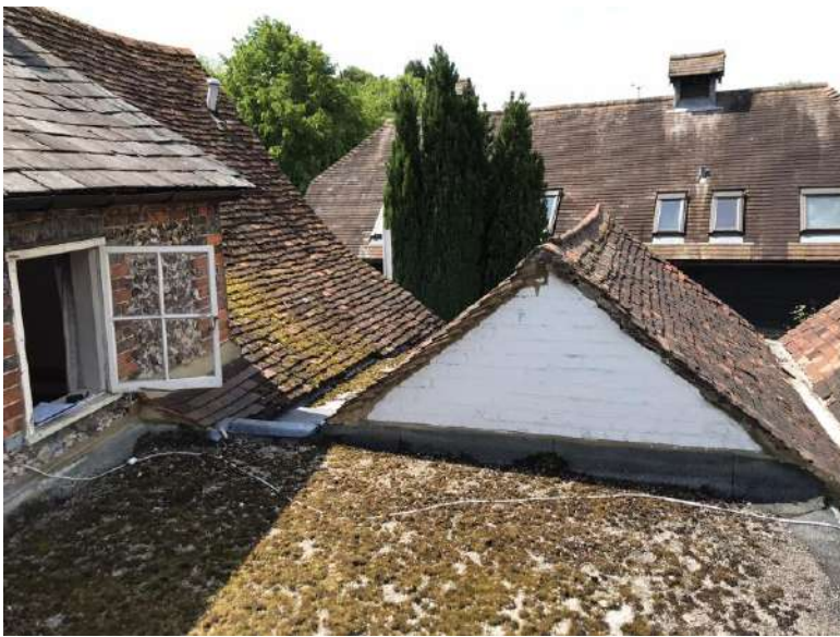
View from the flat roof looking towards no.5 and the dual pitched rear extension abutting the site. The rear extension to no.5 is formed of two dual pitched roofs with lead valley gutters. Also, can be seen the timber side hinged window to the rear of no.7 and the felt flat roof finish
