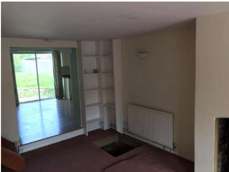
Internal view of lounge to no.7 looking towards the opening to the kitchen and the floor hatch to the cellar. The shelves to the corner are either side of the boxing to the vertical drainage pipe.
