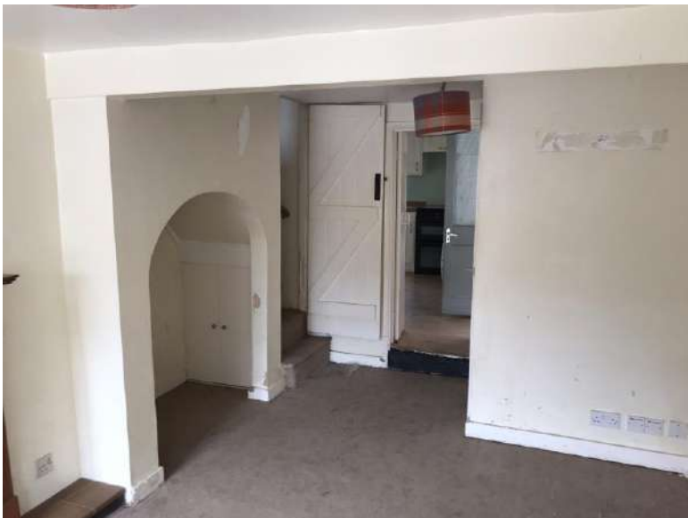
Internal view of the ground floor lounge looking towards an open recess under the staircase. The door to the stair is visible to the centre of the picture, with the wall to the wc to the right. To the background is the opening into the single kitchen straddling both properties
