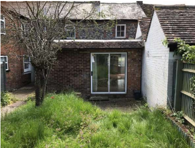
Closer view of the rear extension to the two properties, showing the patio door, tiled mansard roof and brickwork. Also can be seen is the fruit tree and side flanking wall to no.5 and the garden fence.
