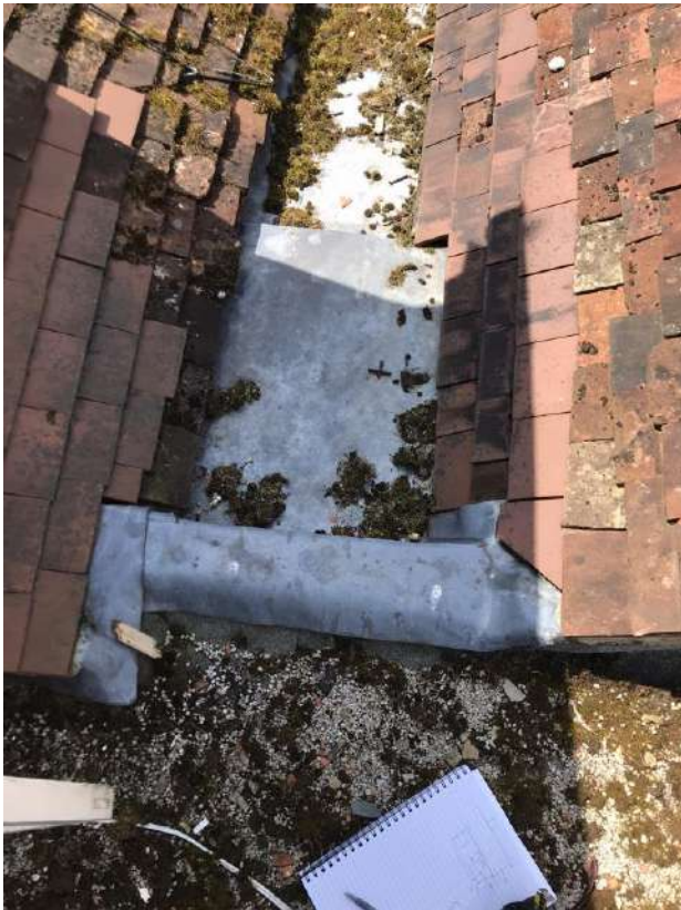
View from the inner lead valley gutter to no.5 where it abuts the felt roof to the site's rear extension.
