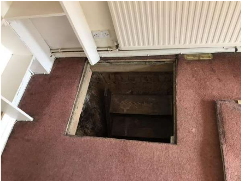
View of the floor opening leading to the steps down to the cellar under no.7
