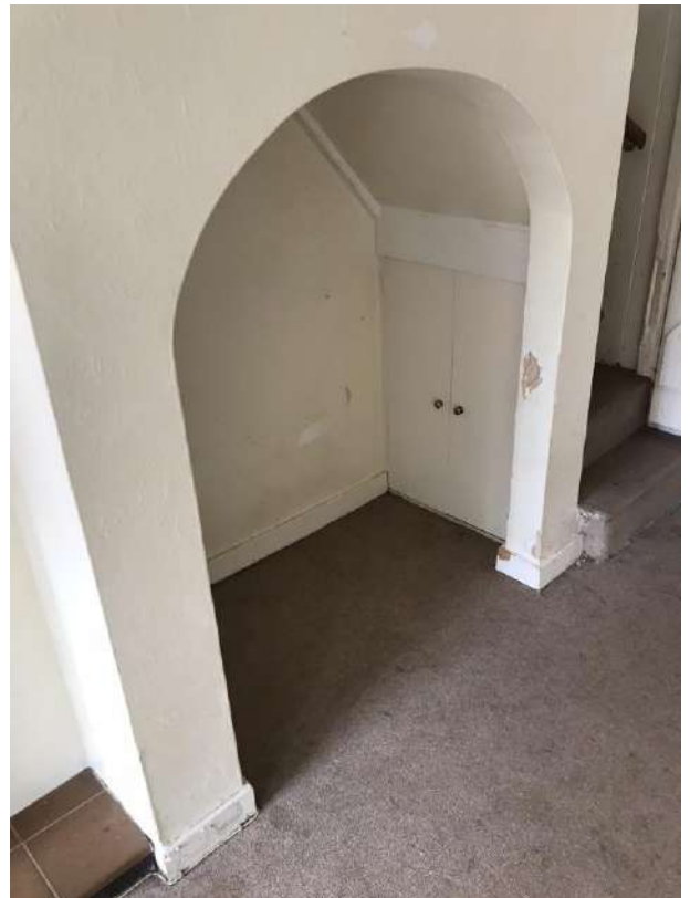
View of the arched opening to the recess under the stairs, with a small storage cupboard under the lower steps
