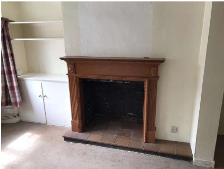
Internal view of the ground floor lounge looking towards the fireplace and chimney stack. The mantelpiece is modern, dating to the 1970s or 1980s. A low level cupboard and shelving, again, a modern addition is visible to the left.
