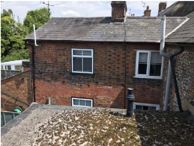
View of the side elevation to the rear of no.11, taken from the roof of the single storey extension to no.7 and 9. The felt roof can be seen and where it laps with the lead flashing that overlaps the tiled mansard roof that runs round the two open eaves. The flue to the boiler to the kitchen extension can be seen projecting through the felt roof.
