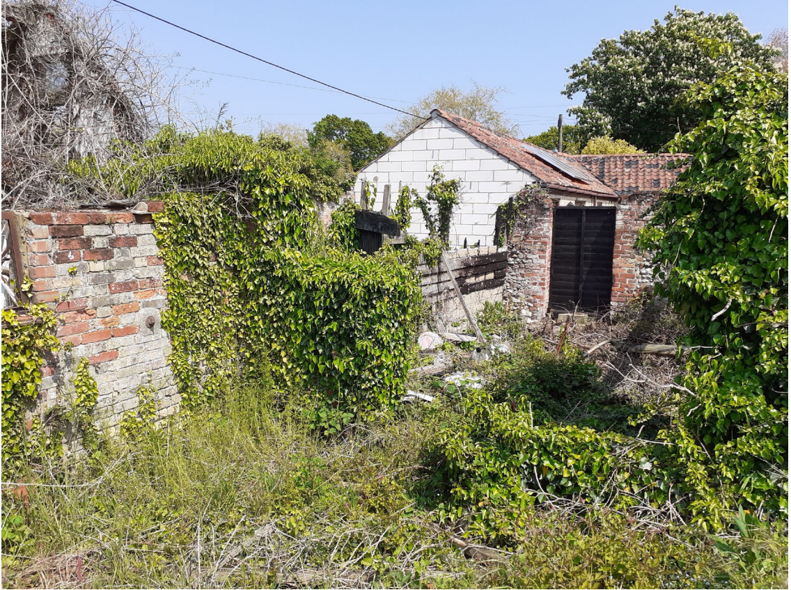
Photograph 7 : Dilapidated barn to the north adjacent to Hall Lane.
