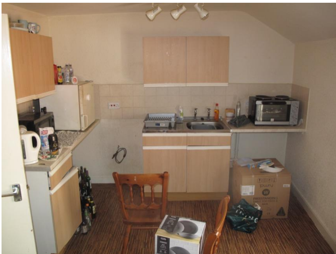
Figure 31 The upper floor of the application property is devoid of historic fixtures or fittings survive. Image courtesy of CSB Architects.
