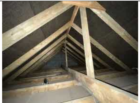
Photo 10. Interior roof space of the pool building showing low height (1m) roofing felt and timbers in excellent condition, affording no access or roosting features for bats
