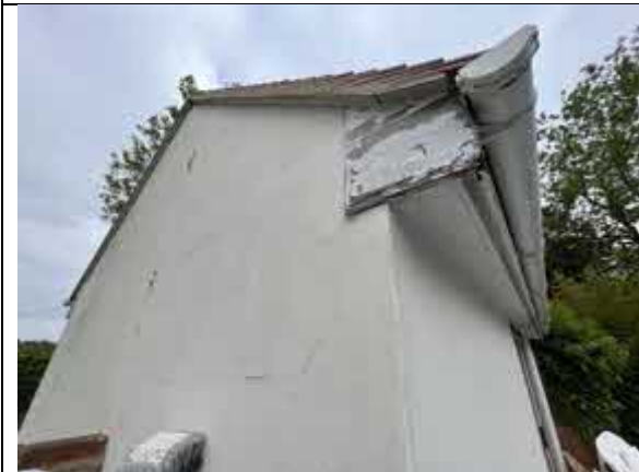
Photo 9. Exterior of pool building showing no cracks or gaps around the soffit box and where the gable wall joins the roof
