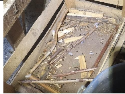
Photo 11: bat droppings beneath internal gable wall.
