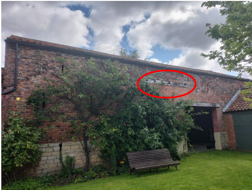
Figure 7. Emergence location 4; Building 2
