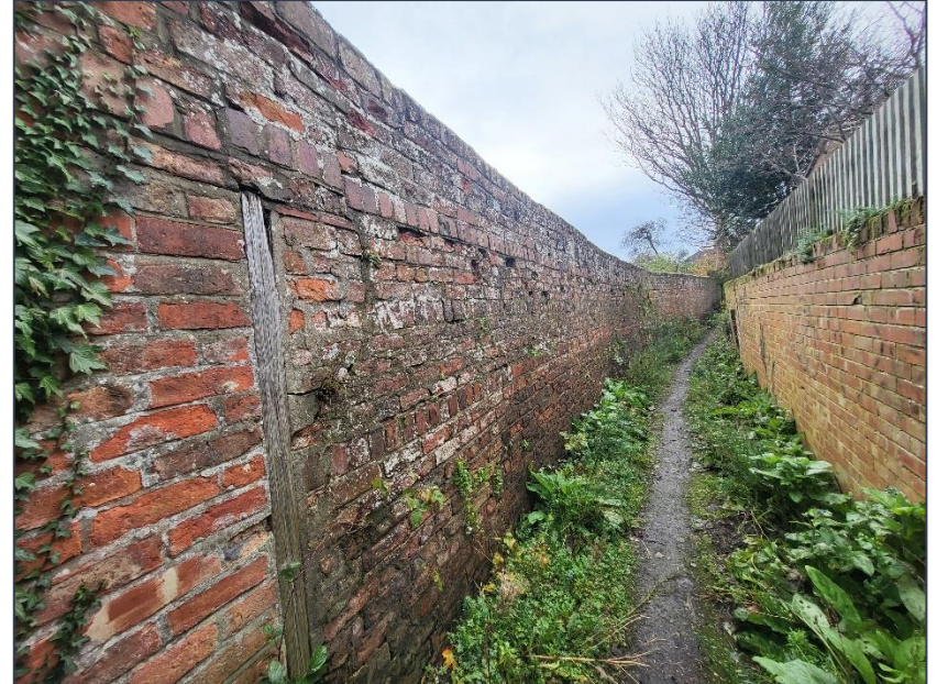
Figure 16 The wall is leaning inwards towards the Site with spalled and damaged brickwork. The wall to the right (engineering brick) has a timber fence to the top.
