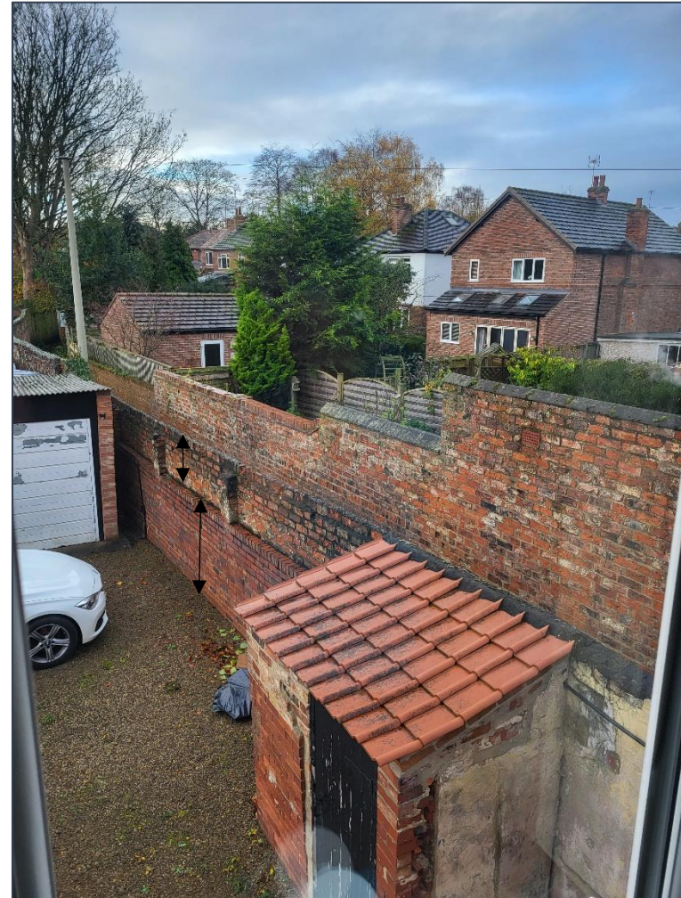
Figure 14 Inside face of boundary wall which has been raised in height several times and an inner skin added in engineering brick.
