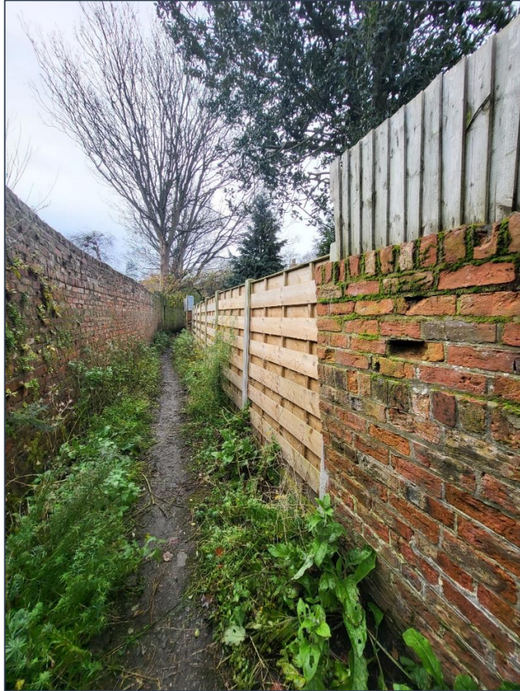
Figure 17 Timber fencing is used further along the lane to the rear of No.3 Greencliffe Drive.
