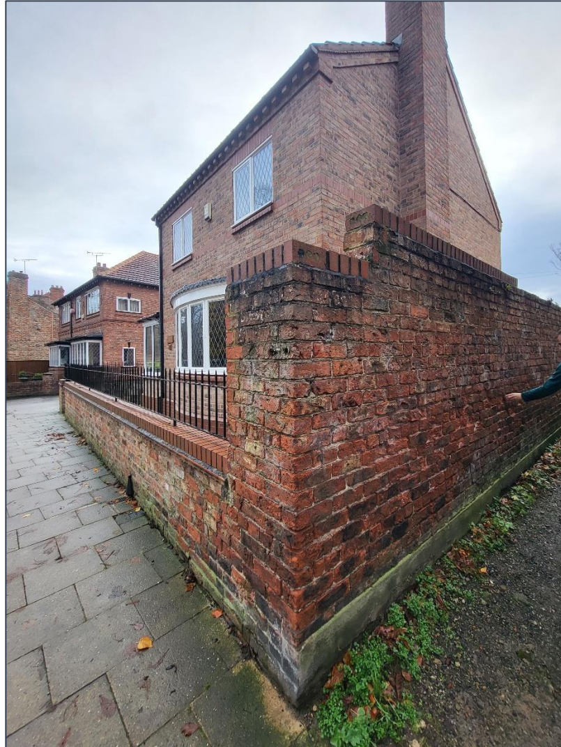
Figure 15 Corner of wall on entry to Love Lane with spalled brickwork, engineering brick cap and cement render to plinth.
