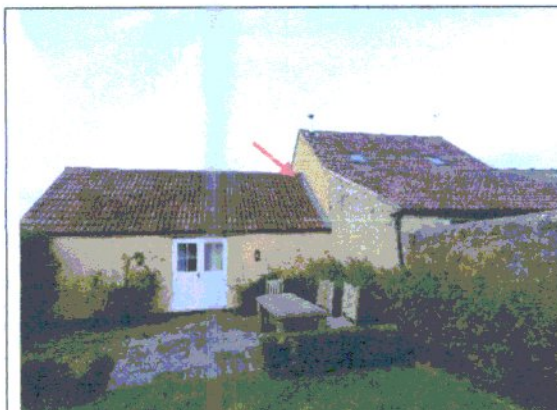
Photo 1: Droppings were found in a cobweb within the roof void at the northern end of a single story extension.
