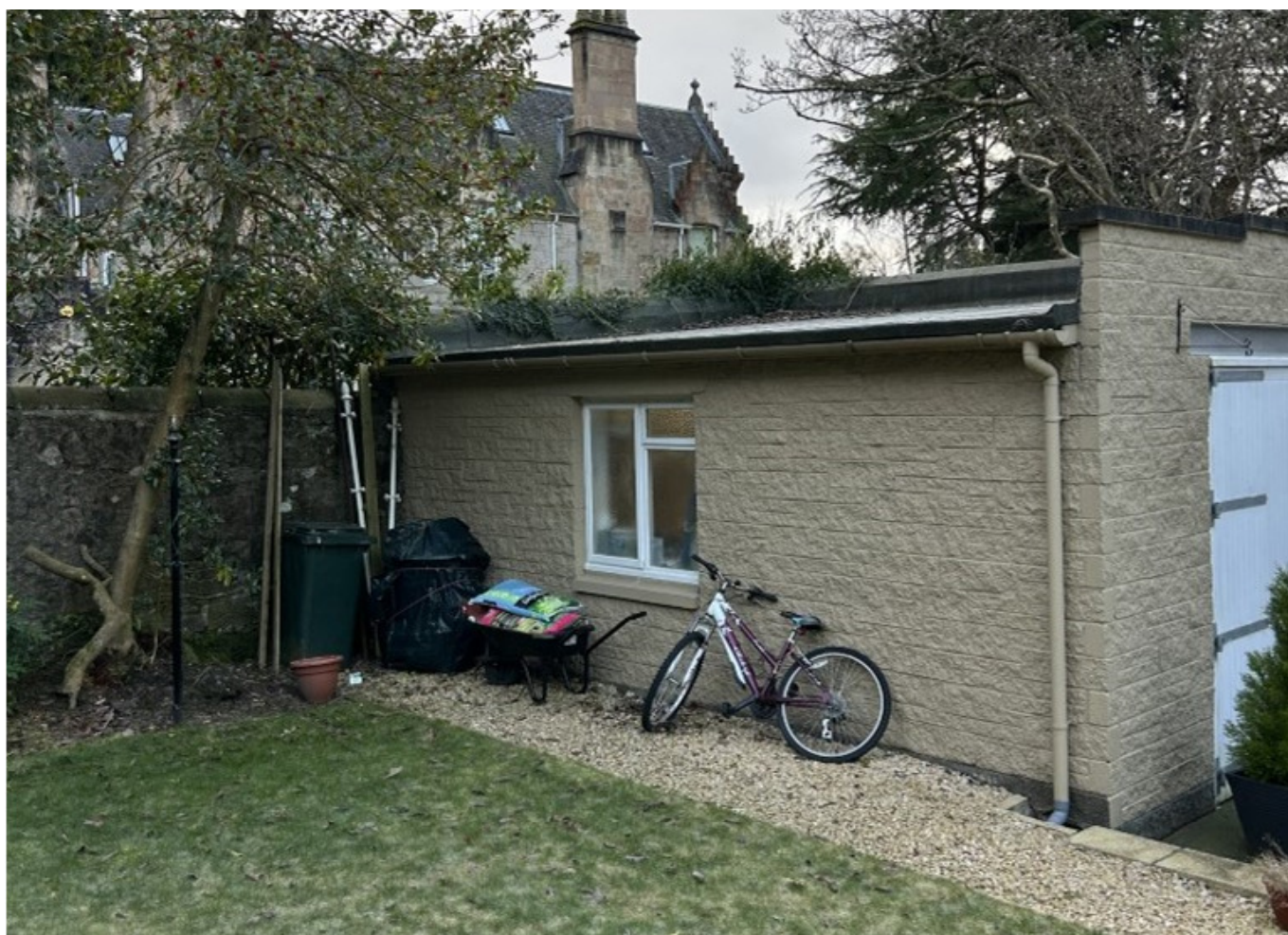
VIEW OF REAR GARAGE WALL - SHOWING NON ORIGINAL WINDOW
