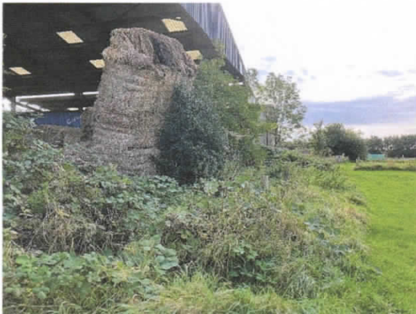
Photo 7: Nettle and bramble dominated margin to rear (west) of Barn 3 (straw bale wall visible)
