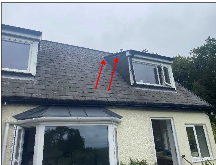
Photograph 7: Gaps underneath the lead flashing
