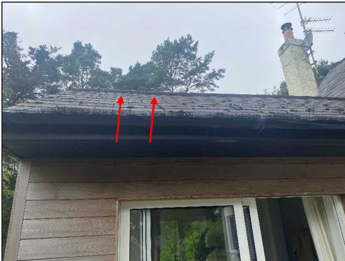
Photograph 6: Gaps underneath ridge tiles
