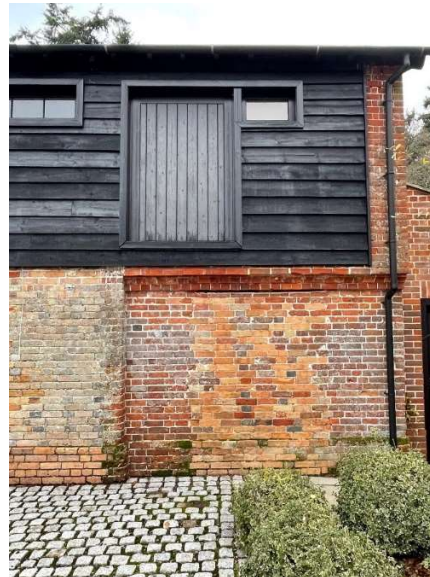
Figure 22 – Evidence of blocked opening to rear elevation
