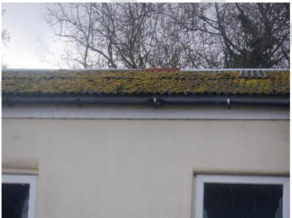
29. Mossy corrugated metal sheeting (B6).
