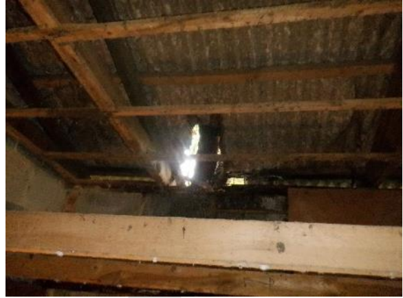
26. Hole in corrugated sheet roofing due to tree branch at the rear corner of the small storage building (B5).
