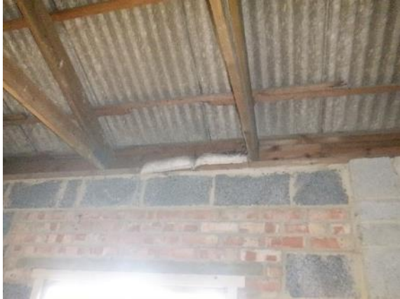
13. Small old birds nest present on the blockwork wall in the open eaves (B1).
