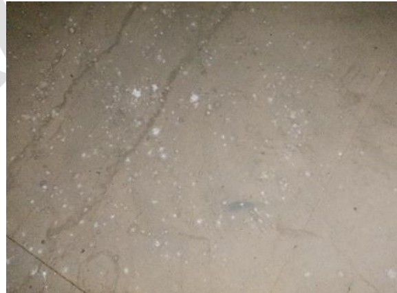
12. Bird droppings present below rafters on raised mezzanine level to the rear of the building (B1).
