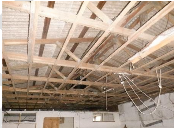
22. Open to the roof internally with an old, raised water tank present (B3).
