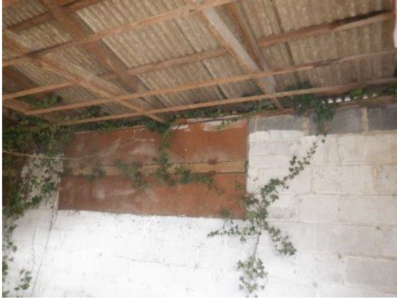
25. Ivy growing over open eaves (B5).
