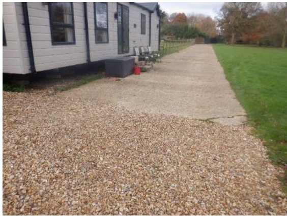
9. Concrete and gravel driveway leading to the north of the site (u1e).
