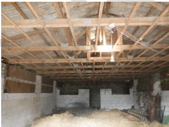
23. Open to the roof internally with an old, raised water tank present (B4).
