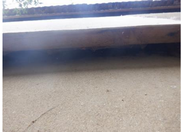
20. The sides of the hay barn featured boarding over old windows, with gaps externally that were very cobwebbed and open internally (B4).
