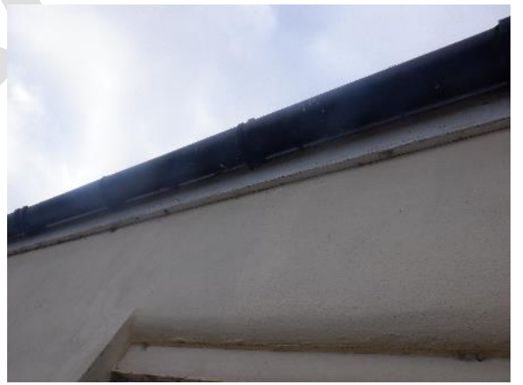
30. Tight timber barge board below the gutter along the eaves (B6).
