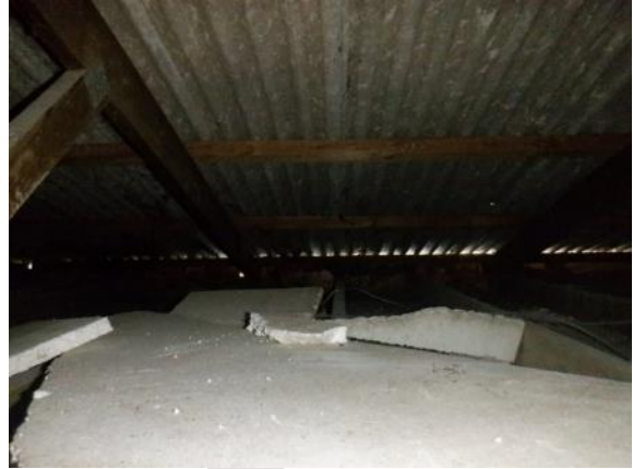
32. Daylight visible at the open eaves (B6).
