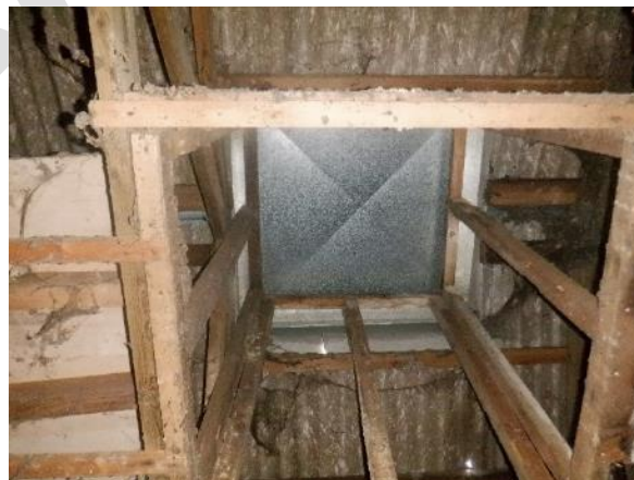
24. Cobwebbed throughout rafters and around raised vent (B3).
