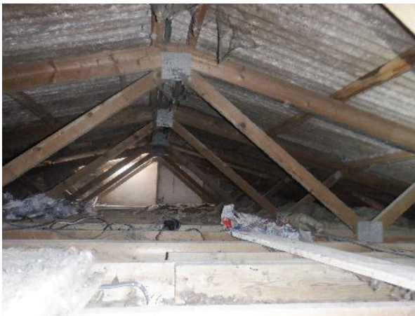
33. Boarded northern gable, with daylight visible and fibreglass insulation present below wall (B6).
