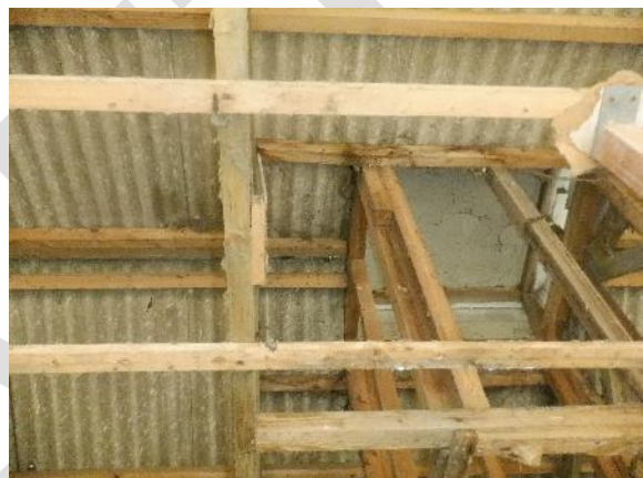
16. The rafters and ridge were heavily cobwebbed throughout (B2).
