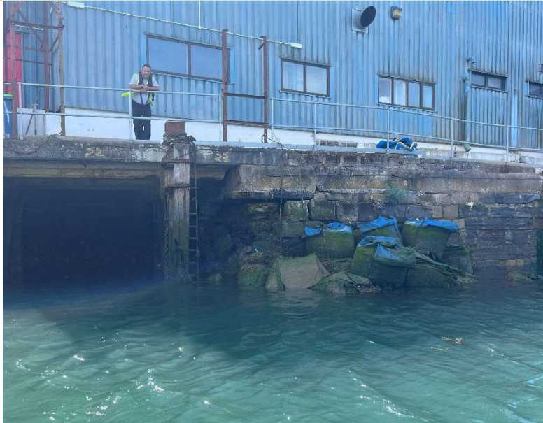
Sea wall requiring repairs/reinstating
