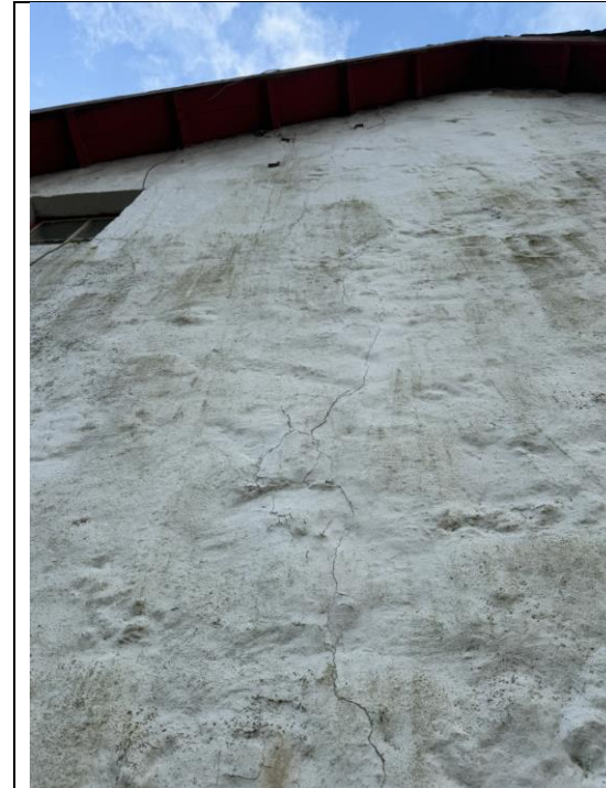
Figure 24 External gable wall showing evidence of minor cracking to the external finishes.
