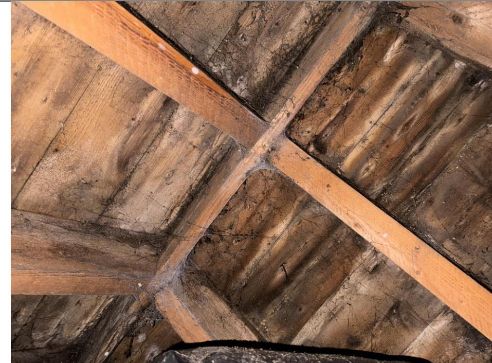
Figure 9 Inside main farm building roof space. Showing signs of water ingress and rot
