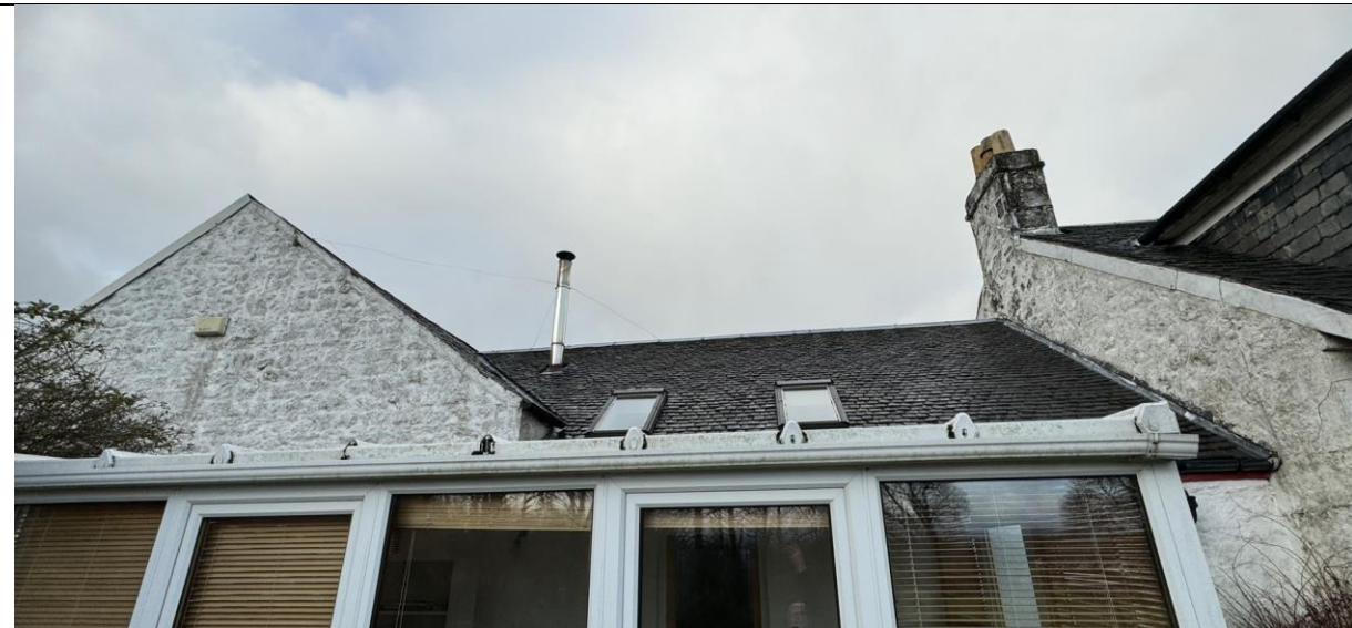
Figure 8 Images of external roof from rear showing slate covering, rooflights and metalworks
