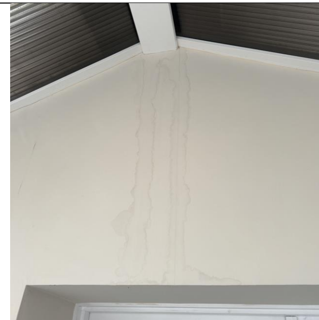
Figure 21 interface between conservatory and main building showing signs of water ingress
