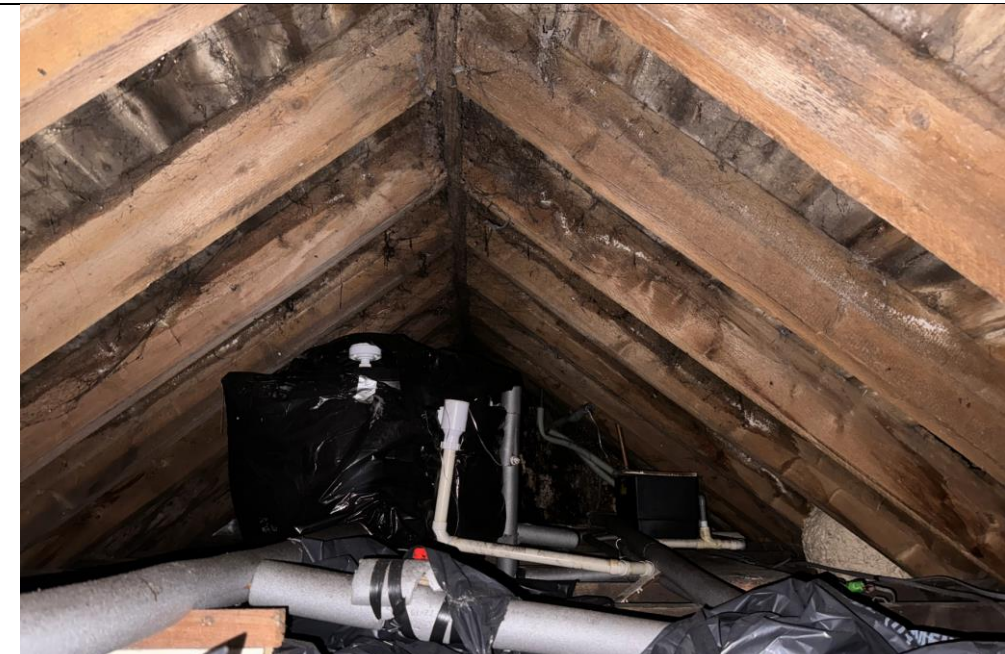
Figure 10 Inside main farm building roof space. Showing signs of water ingress and rot
