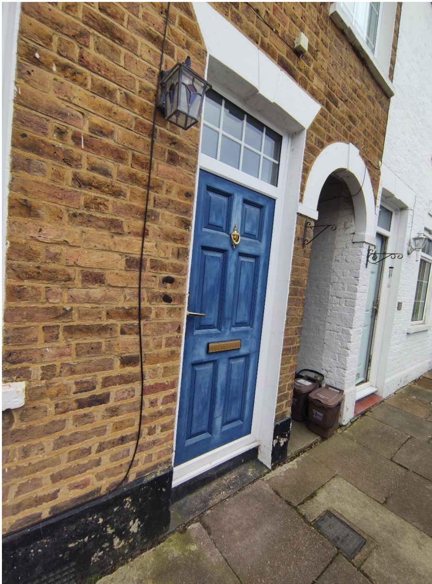
Front access door:
