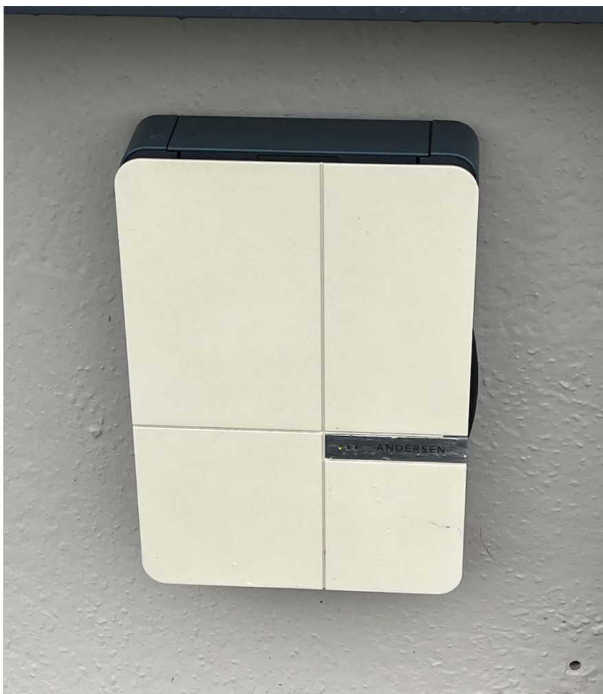
Annex 3: Photograph of EV charging point
